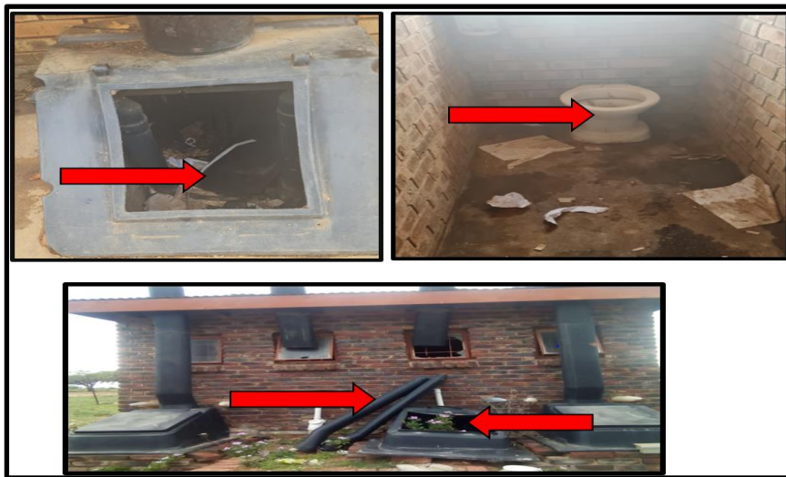
Figure 3.1: Damaged drying plate, inspection cover, and ventilated pipe and broken toilet lid
