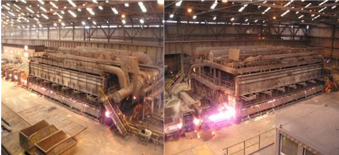
Figure 4-5: Mill 4 reheating furnace
