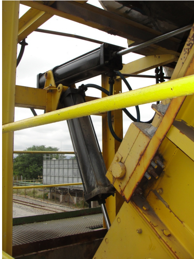
Figure 66 – Pneumatically operated loading box door on surface silo at Mine D
