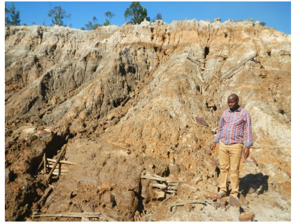
b) Erosion gullies on the sides of the tailing dump.
