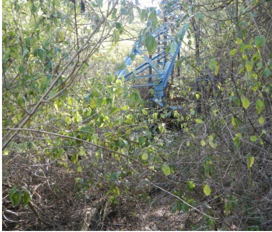
c) Neglected steel structures.
