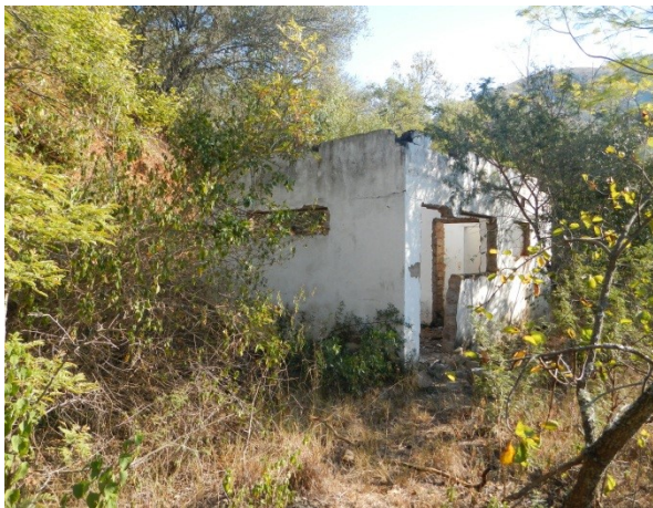
a) Dilapidated mine building.
