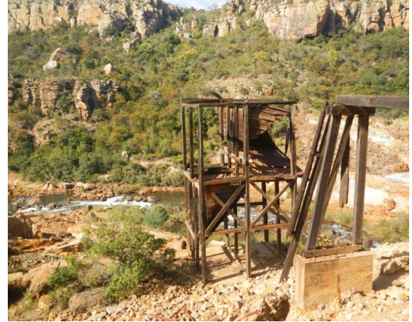
b) Steel structure used for conveyor system.
