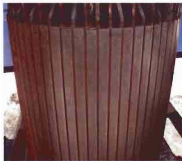
Photo 7.1 The MCFR iron core in excellent condition after running on load for 1.8 years
