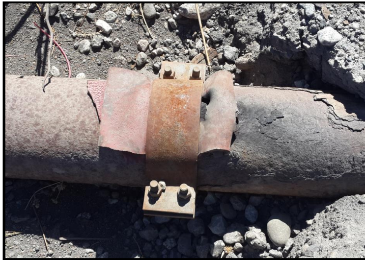
Figure 46: A punch leak in a compressed air network
