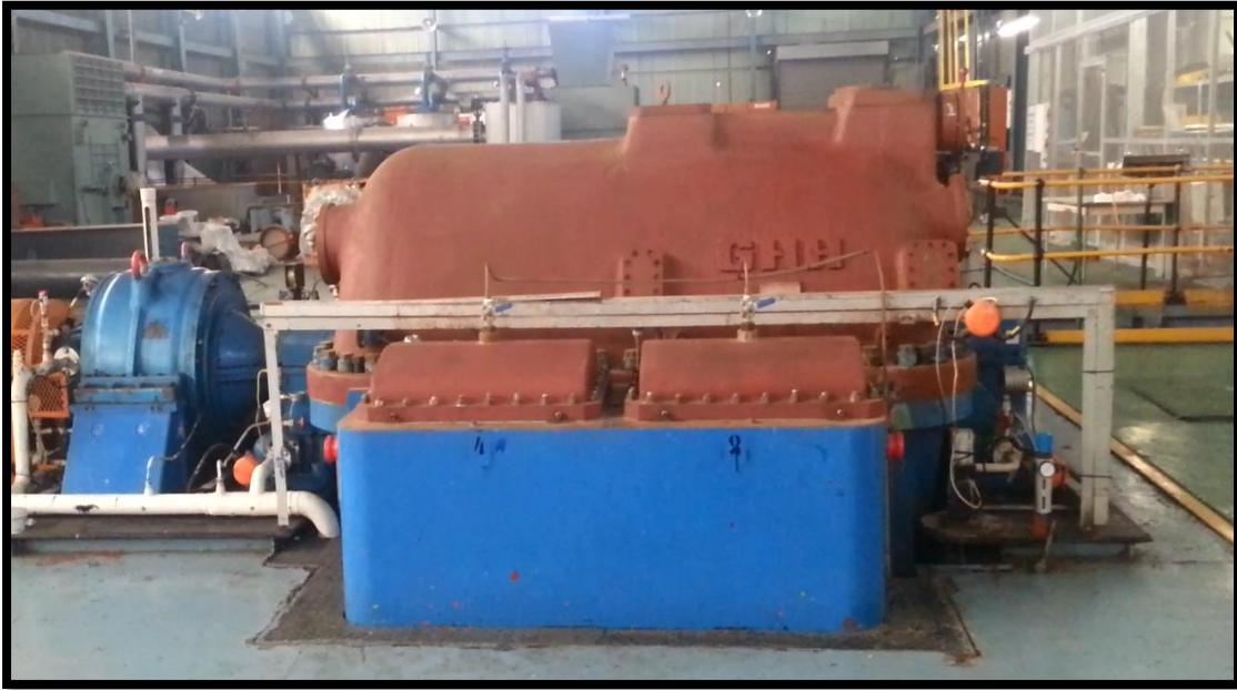
Centrifugal compressor installed on a platinum mine
