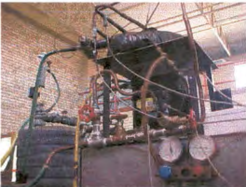
Photo 3: Compressor and Condenser (top) mounted on top of environmental chamber.
