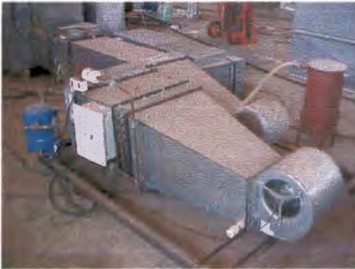
Photo 2: Air Controller: heating elements (far), cooling coil (front) and humidifier.
