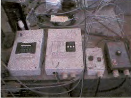
Photo 7: Environmental chamber controls: fan speed, heaters & humidifier.
