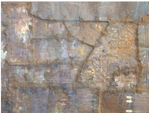
Fig. 2.31. Close-up of rust fragments stitched together to form a surface.
