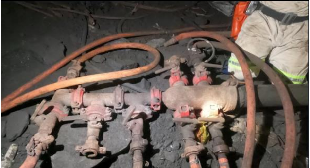
Figure 58: Compressed air manifold modified to supply eight hoses 17
