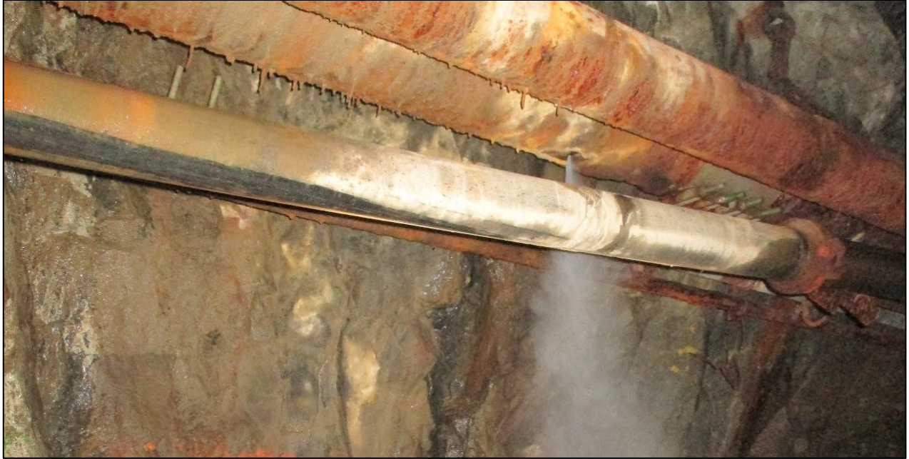
Figure 12: Example of unintentional wastage: Pipe leakage due to corrosion 6
