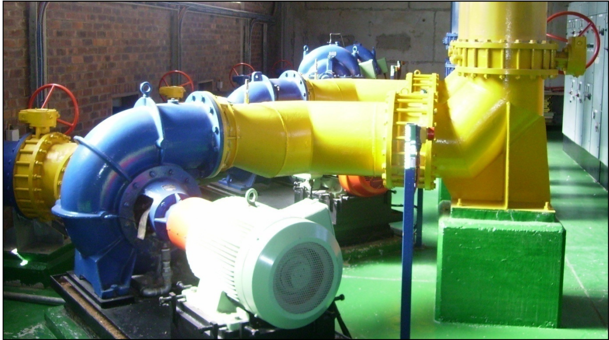
Figure 31: Mine A - transfer and pre-cool supply pumps and valves
