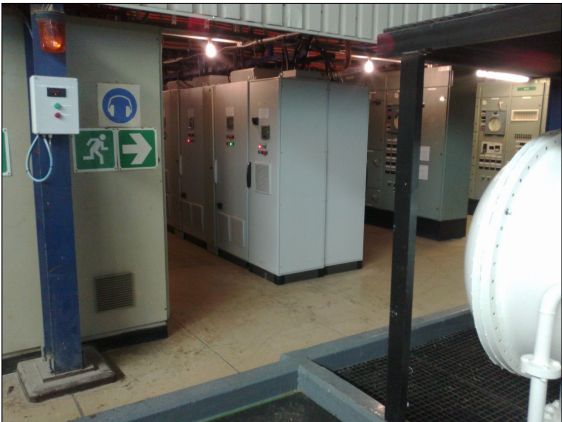
Figure 25: Mine A - installed BAC, evaporator and condenser VSDs (1)
