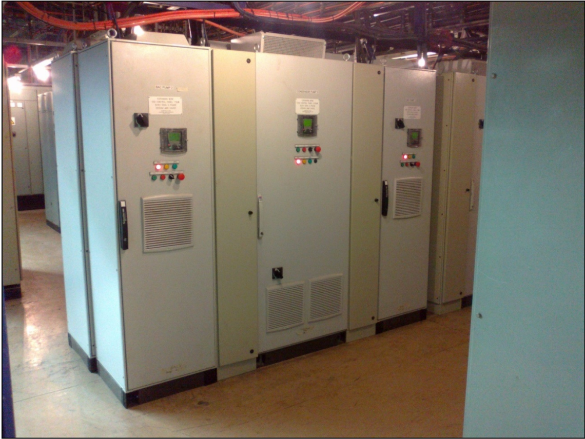
Figure 26: Mine A - installed BAC, evaporator and condenser VSDs (2)
