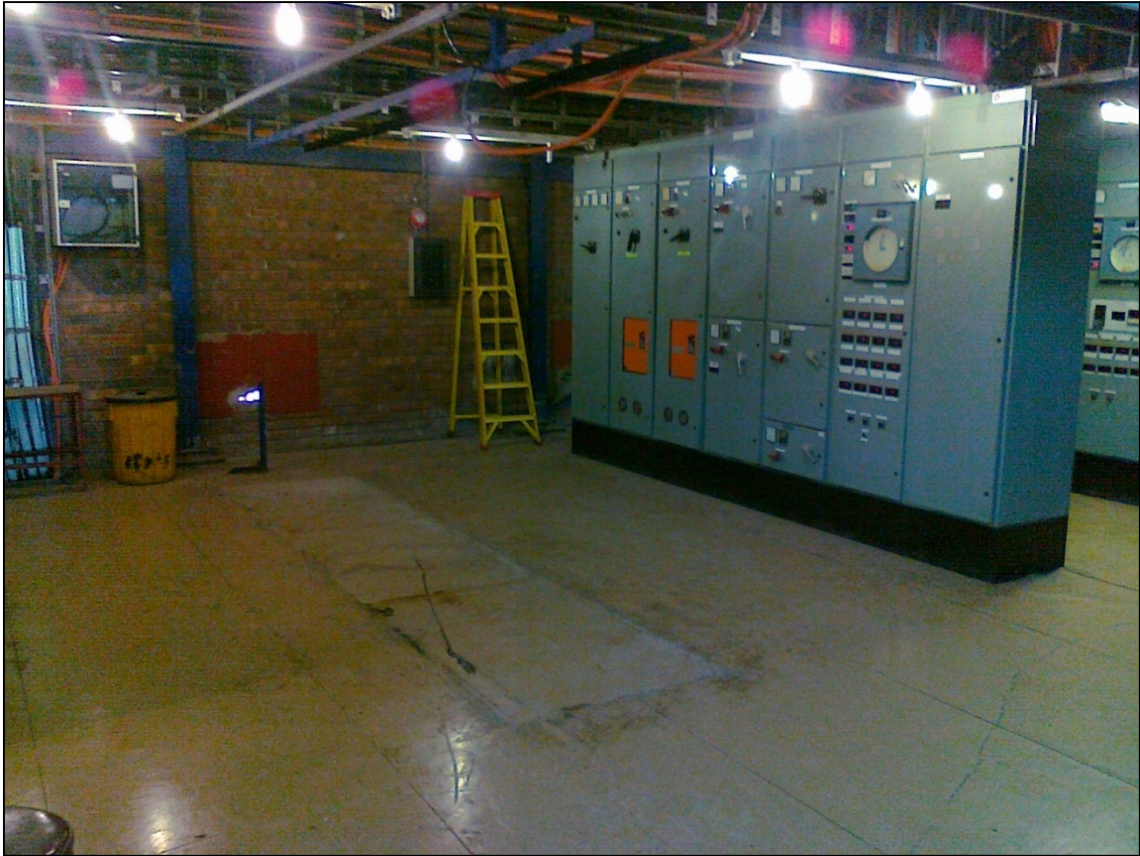
Figure 24: Mine A - location where VSDs will be installed
