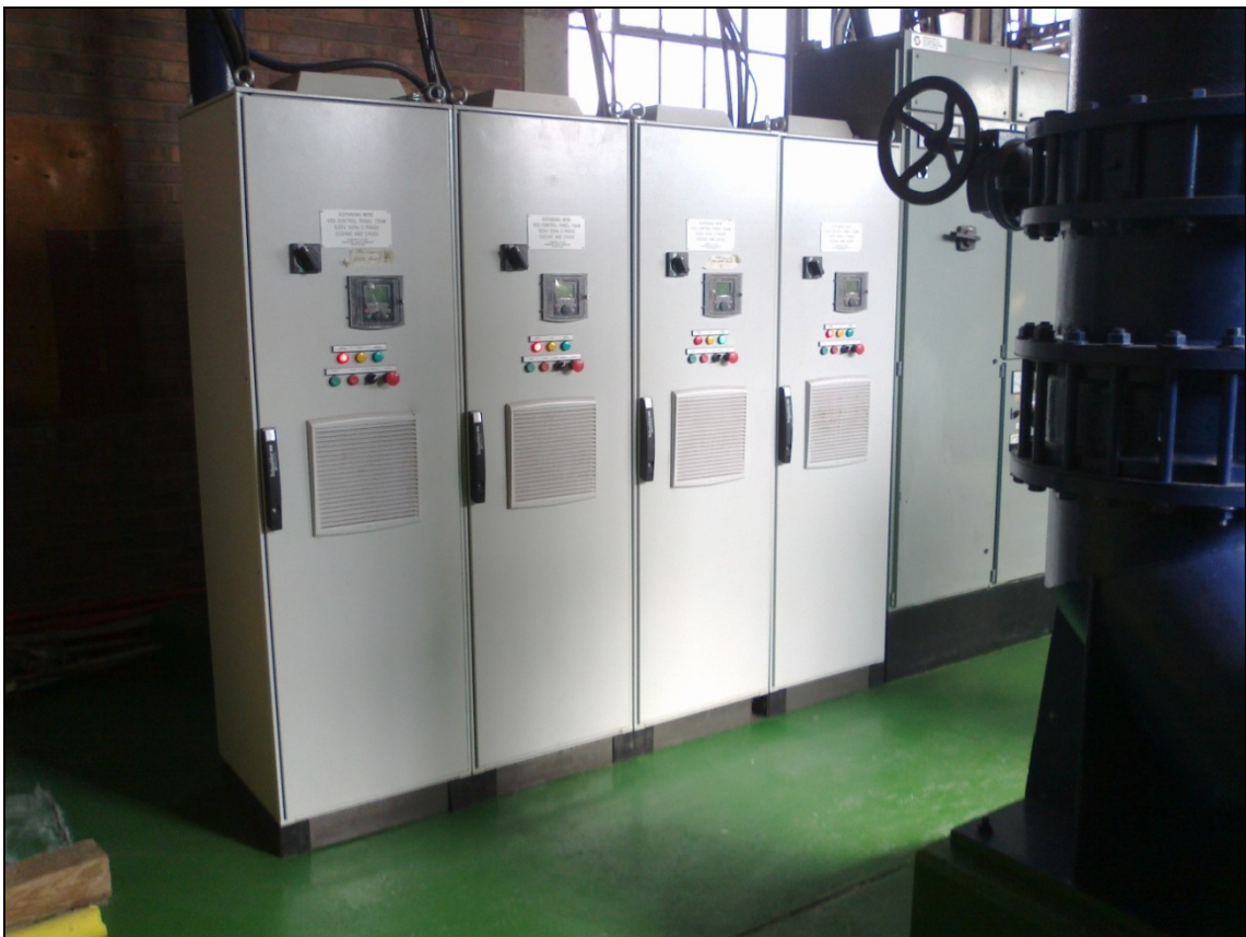
Figure 27: Mine A - pre-cooling feed and transfer pump VSDs
