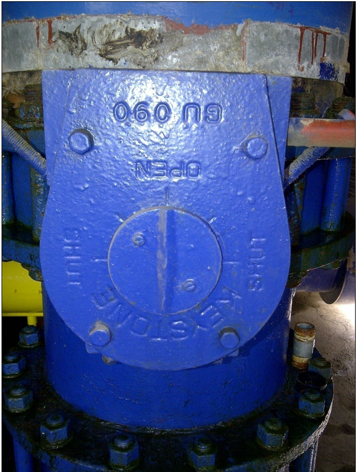
Figure 28: Mine A - BAC flow calibration valve
