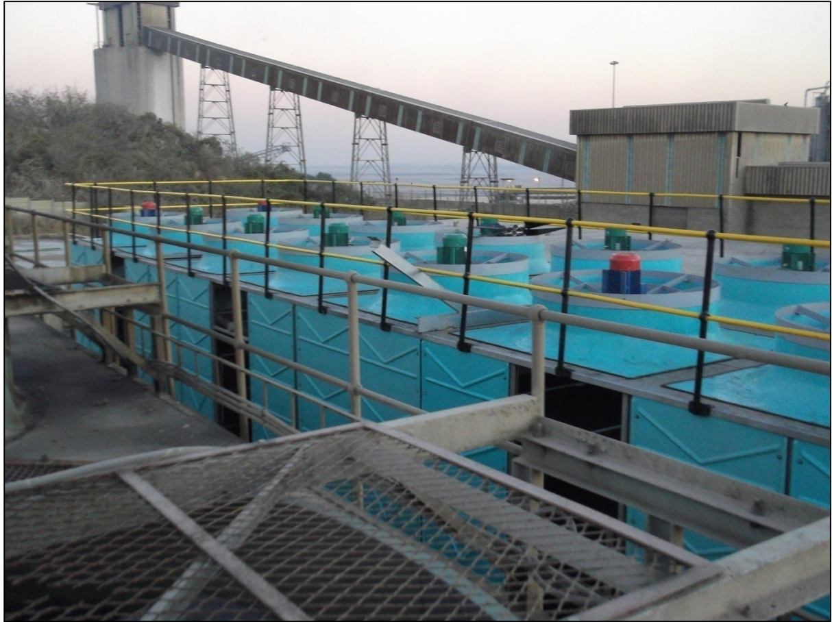
Figure 41: Mine B - new pre-cooling towers bank 1
