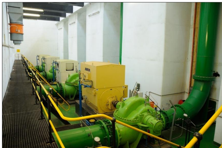
Figure 39: Grootfontein pump station
