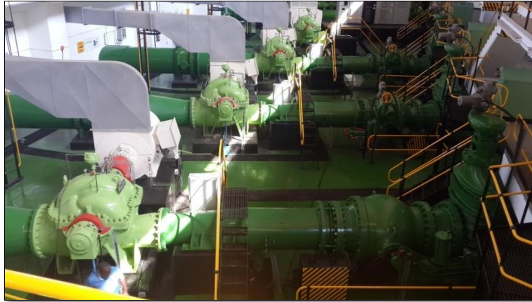
Figure 30: Grootdraai pump station
