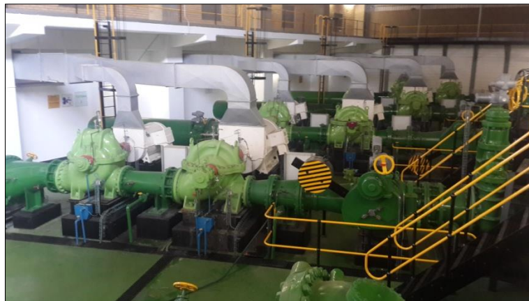
Figure 34: Tutuka pump station
