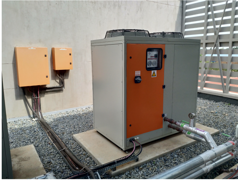
FIGURE 3.3: One of the 90 [kW] ASHP units of the system.
