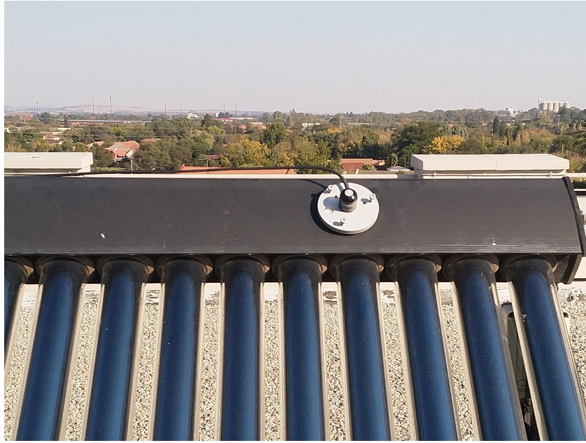
FIGURE 3.7: The pyranometer installed on the SWH bank.
