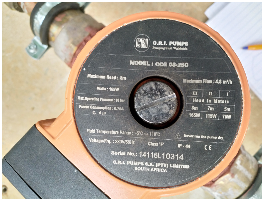
FIGURE J.1: Solar water heater circulating pump
