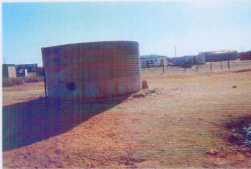
Picture 3: A non-functioning water service
