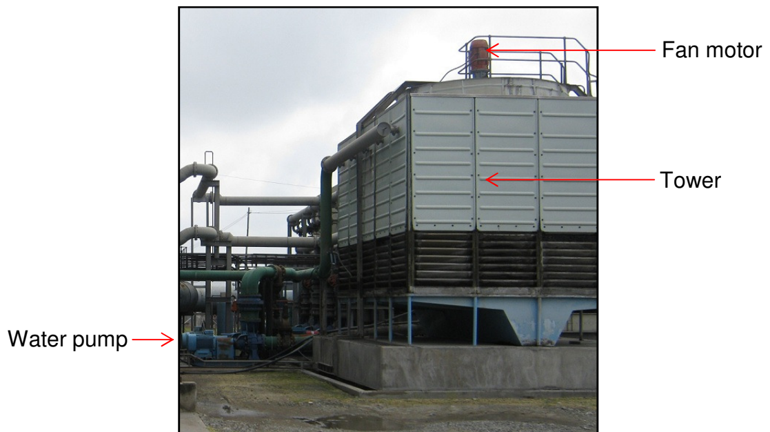
Figure 3: Compressor cooling tower
