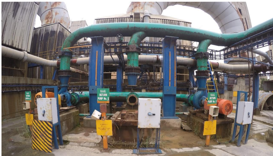
Figure 4-20: Existing BAC return pumps
