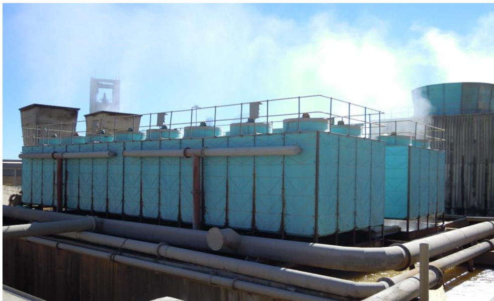
Figure 4-13: New precooling towers
