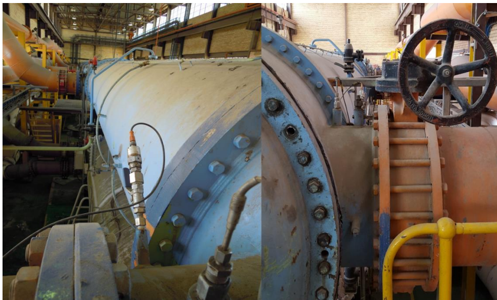
Figure 4-7: Condenser water thermocouple
