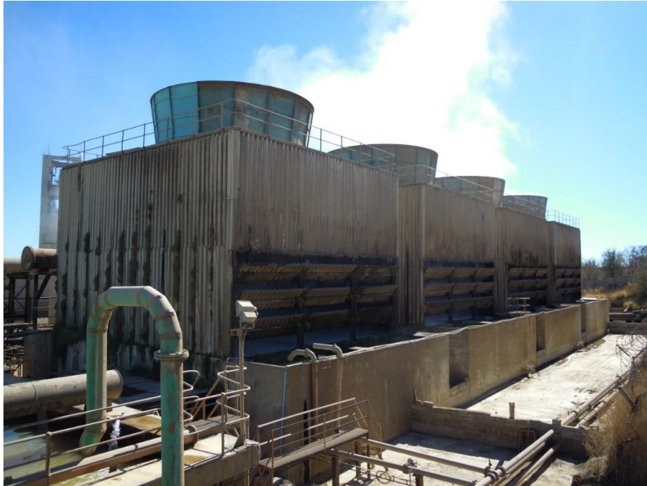
Figure 4-6: Condenser cooling towers
