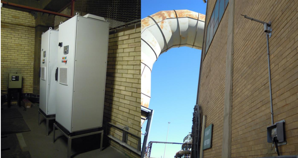
Figure 4-10: BAC return pump VSDs and Testo weather station
