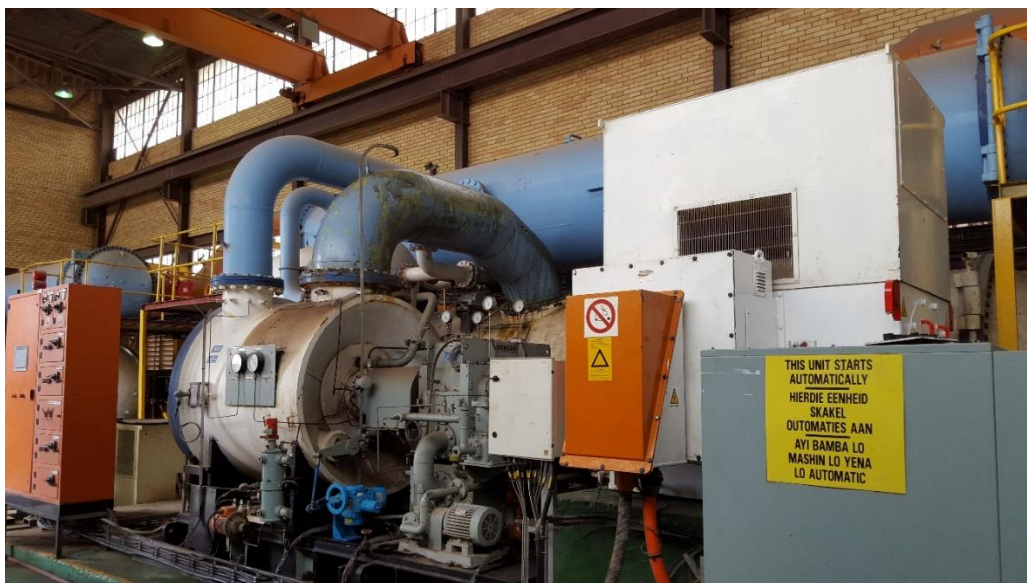
Figure 4-15: Refrigeration machine no. 2
