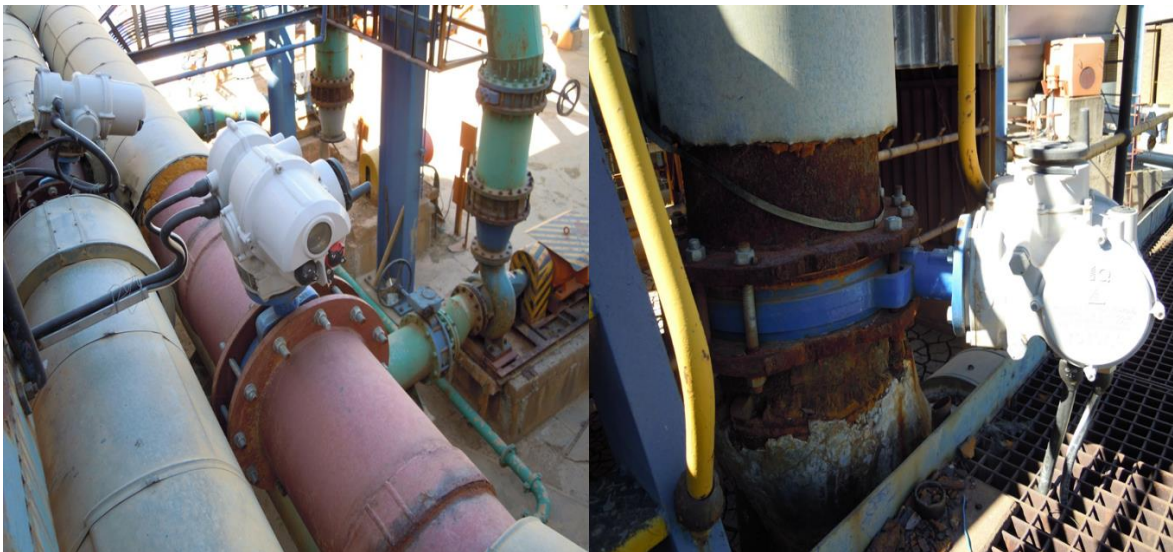
Figure 4-11: BAC water supply control valves
