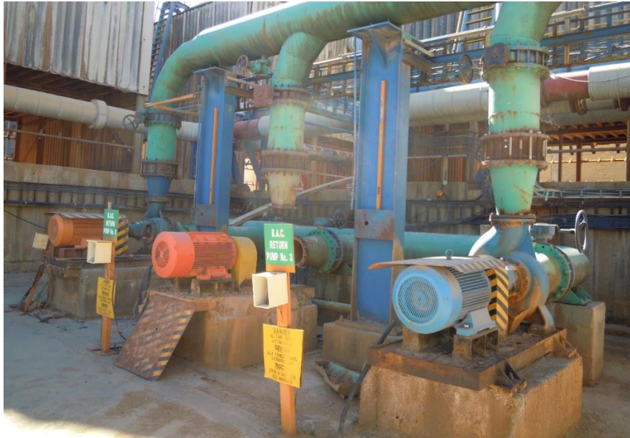
Figure 4-8: BAC return pumps
