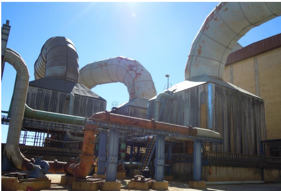
Figure 4-9: BACs with BAC sumps
