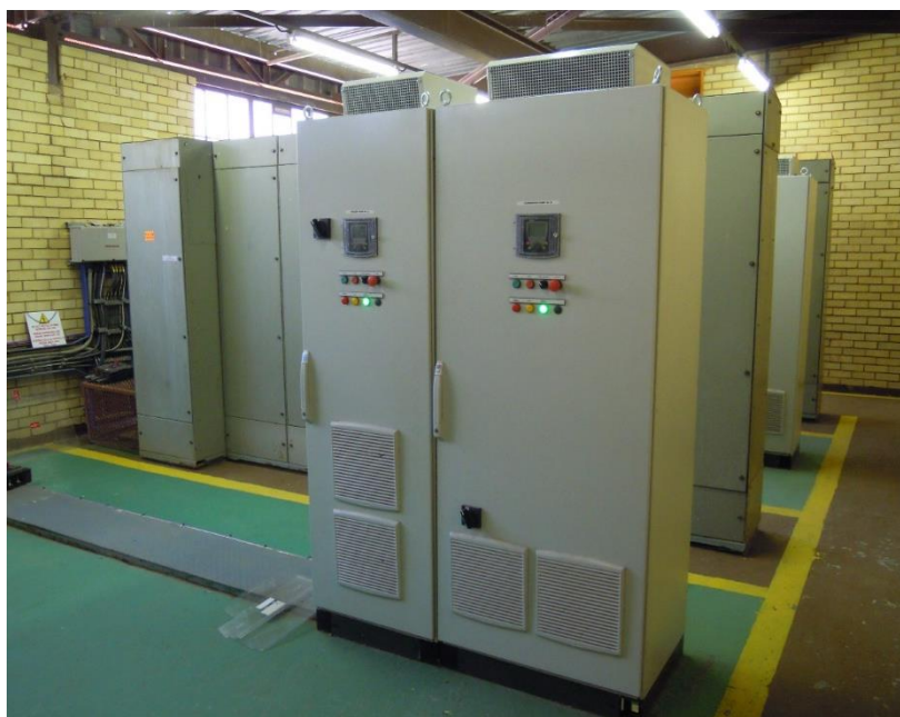
Figure 4-4: Evaporator VSD and condenser VSD
