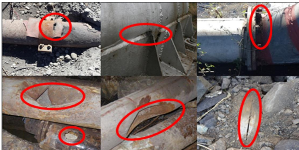
Figure 34: Examples of air leaks on mining compressed air reticulation networks 16
