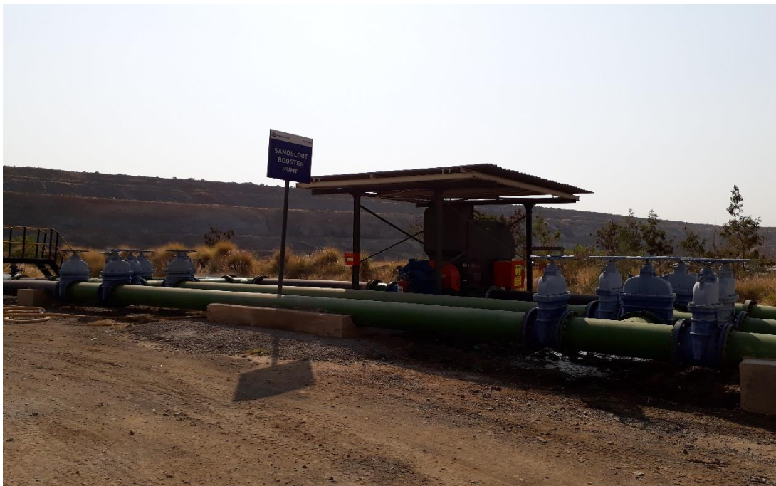
Figure 38: Sandsloot booster pump station
