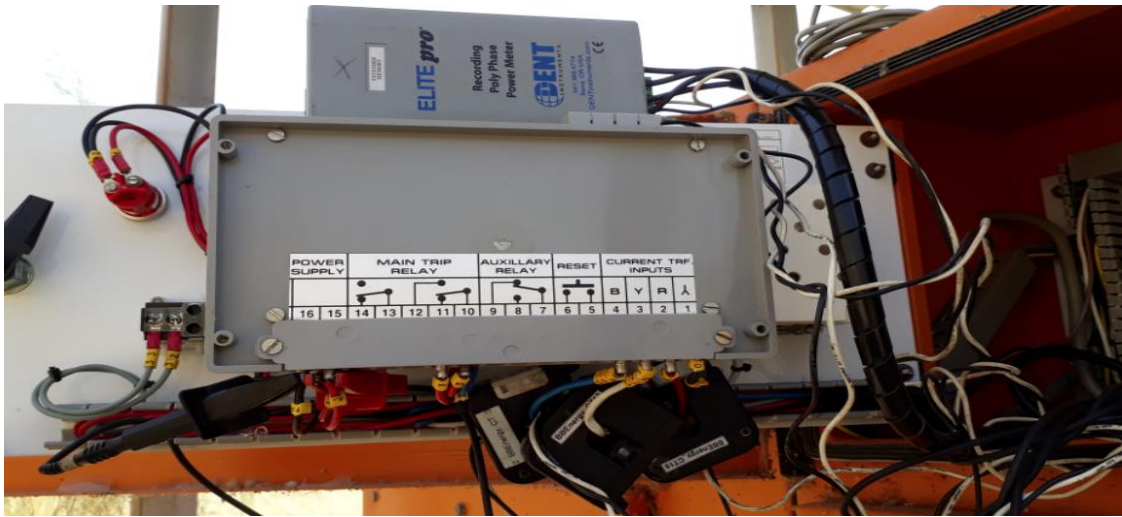
Figure 37: Installation of Dent ElitePro Recording Poly Phase Power Meter
