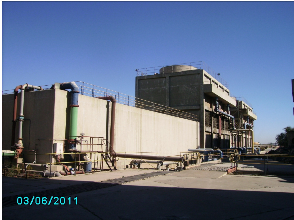
Figure 10: Mine A - surge dam and pre-cool towers
