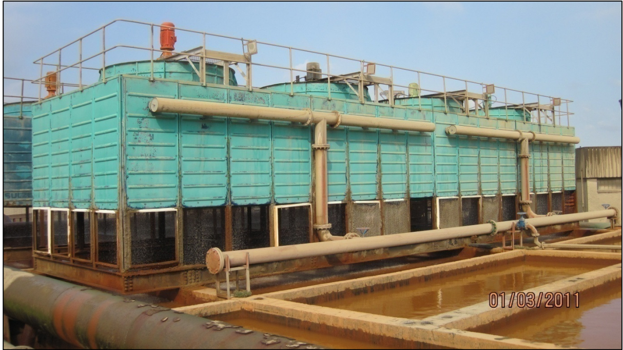
Figure 17: Mine B - existing pre-cooling towers (1)
