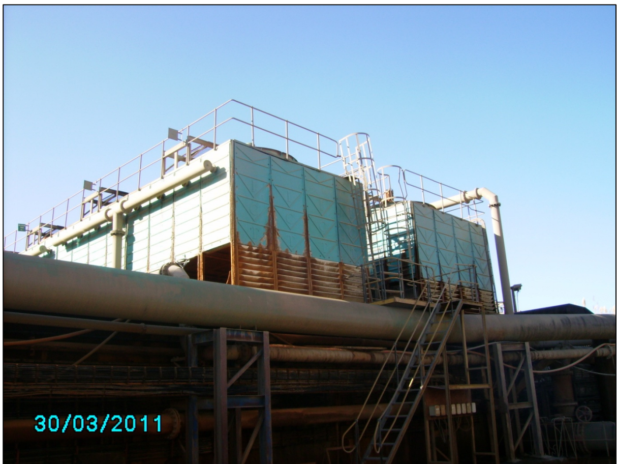
Figure 18: Mine B - existing pre-cooling towers (2)
