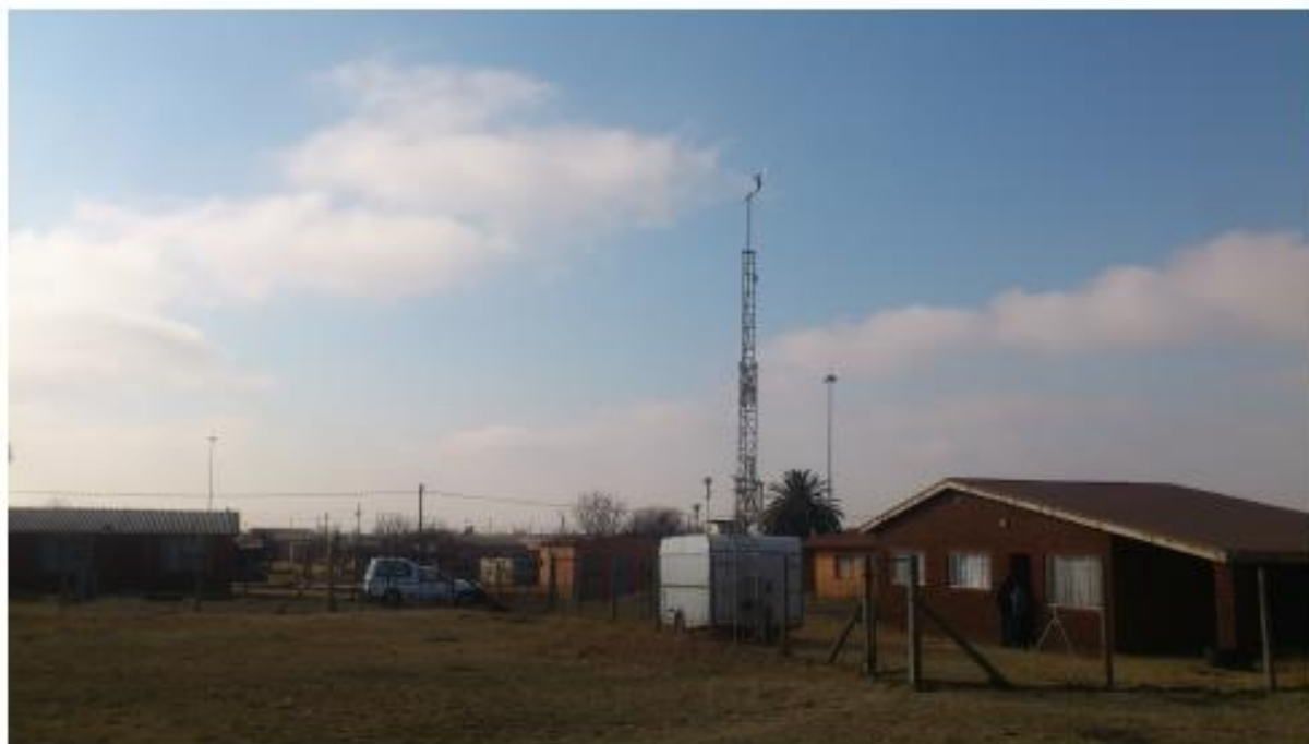
Figure 3-25. The mobile monitoring station where the bulk of the ambient air quality measurements were made
