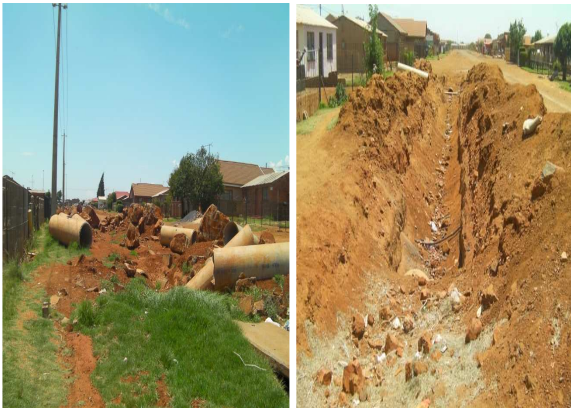
Picture 5.3 Incomplete storm-water drainage system
