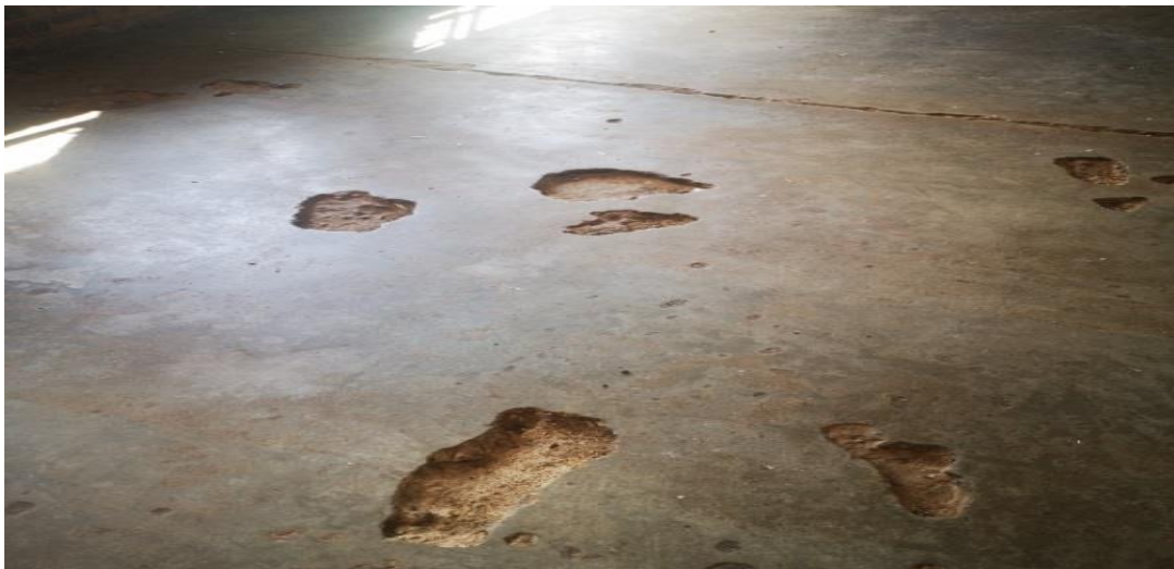
Figure 6-15: Potholes on floors
