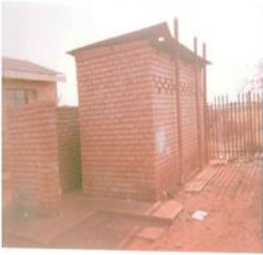
Figure 6-24: Poorly maintained toilet
