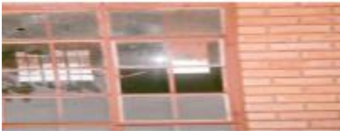
Figure 6-14: Broken windows in a classroom
