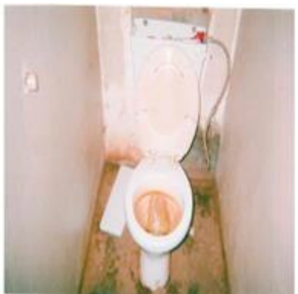
Figure 6-23: Poorly maintained toilet
