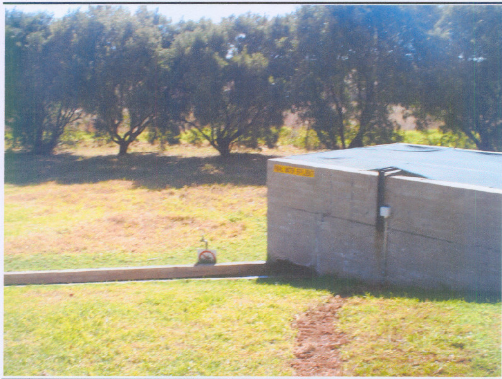
Welverdiend Chlorination Channel and Discharge Point
