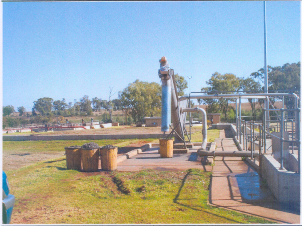
Figure 19 Khutsong - Grit Removal
