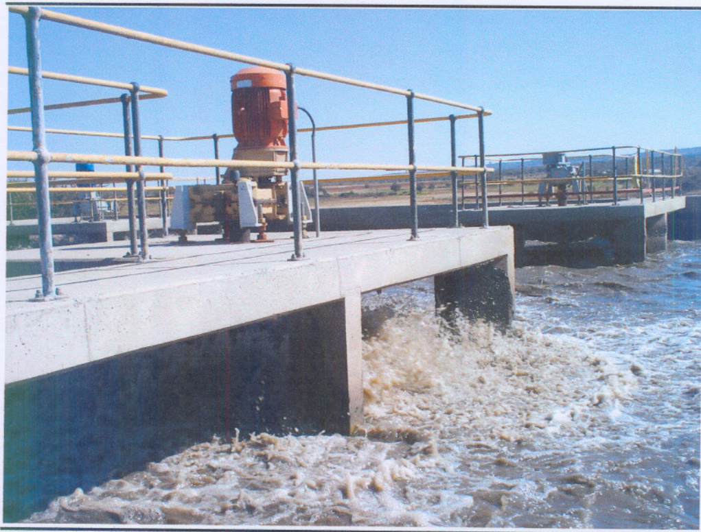
Figure 9 Wedela Aeration Chamber
