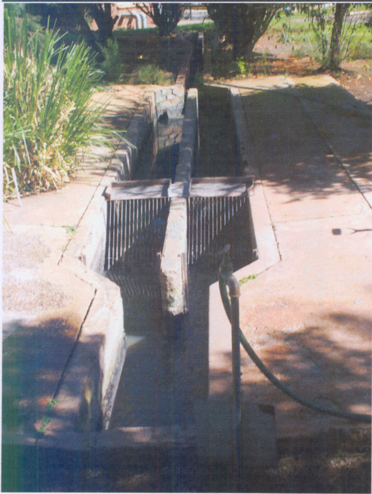
Weloverdiend - Inlet Works
