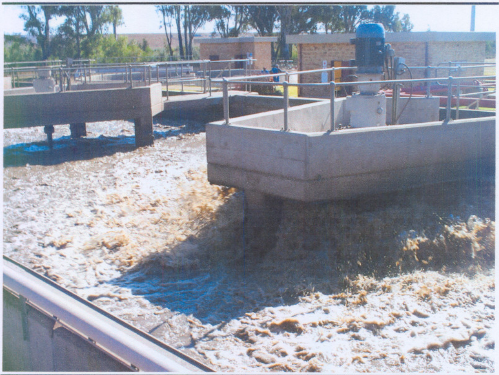
Figure 20 Khutsong Aeration Chamber
