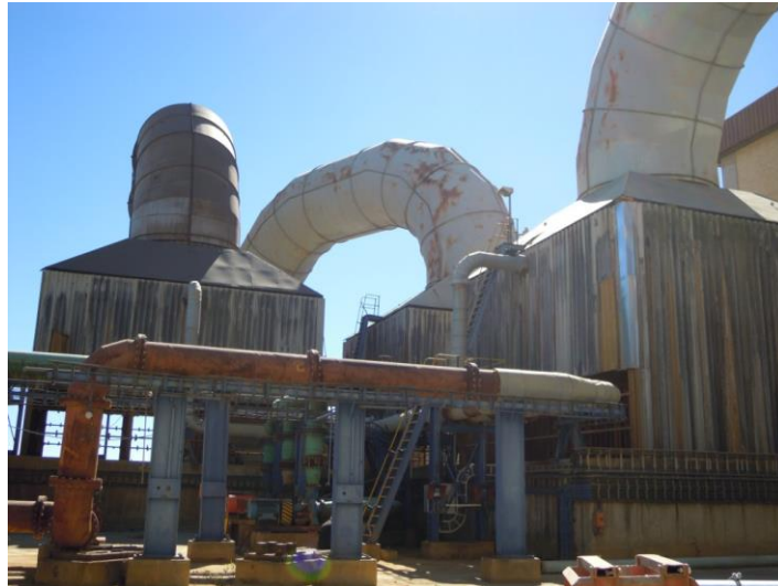
Figure 36: Three BACs currently in operation at the mine
