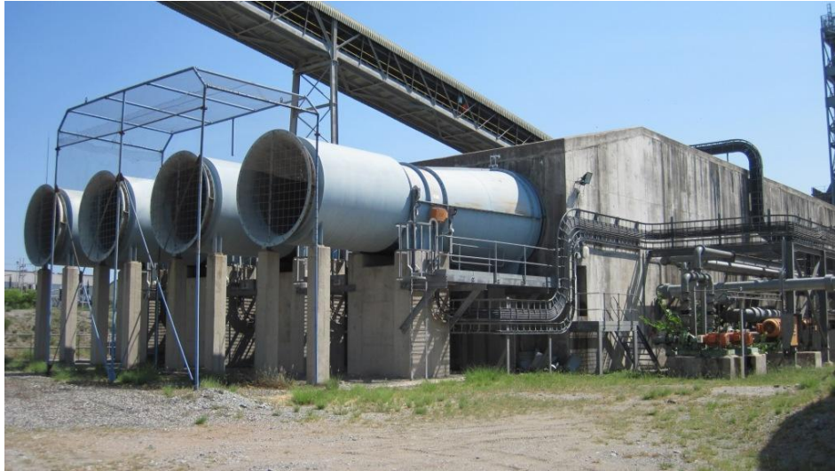
Figure 18: A horizontal spray chamber BAC installed on a platinum mine near Thabazimbi
