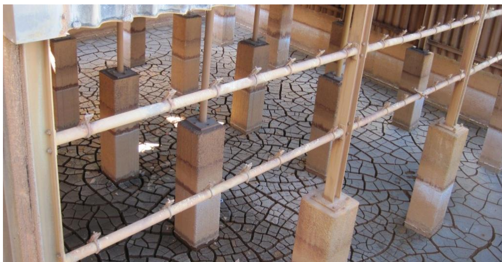
Figure 40: Sediment build up in BAC sump
