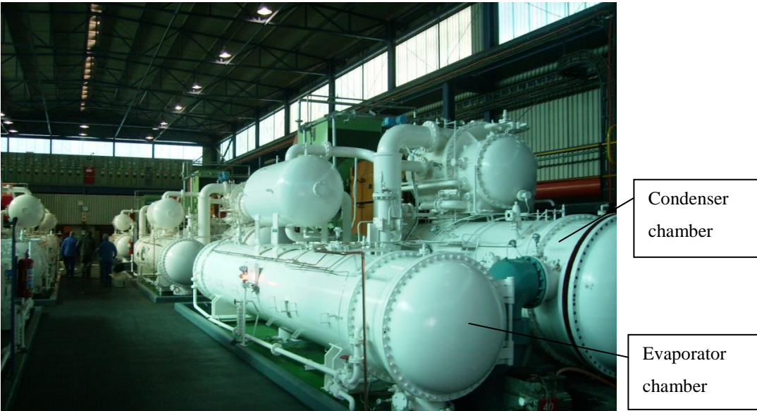
Figure 6: Shell and tube heat exchanger chillers typically used at a gold mine
