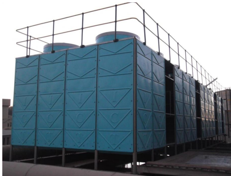
Figure 34: Pre-cooling towers currently in use at the mine
