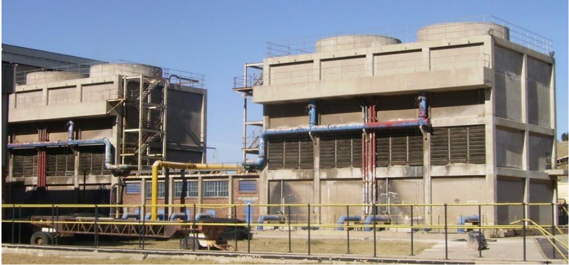
Figure 13: Example of pre-cooling towers typically used on mines
