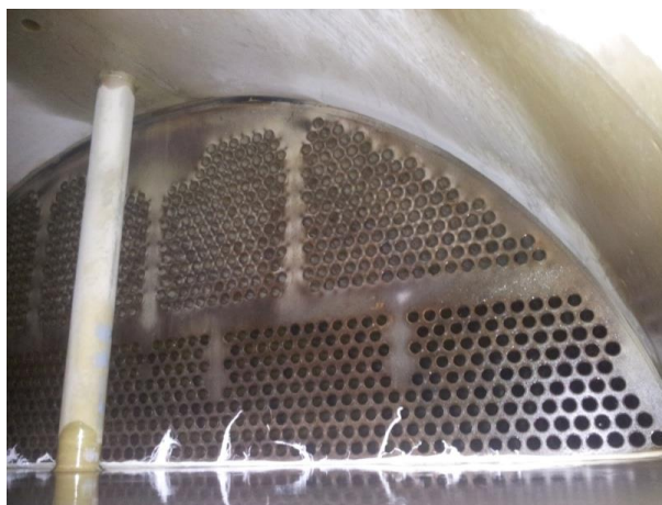
Figure 38: Heat exchanger tubes within the evaporator chamber of the chiller
