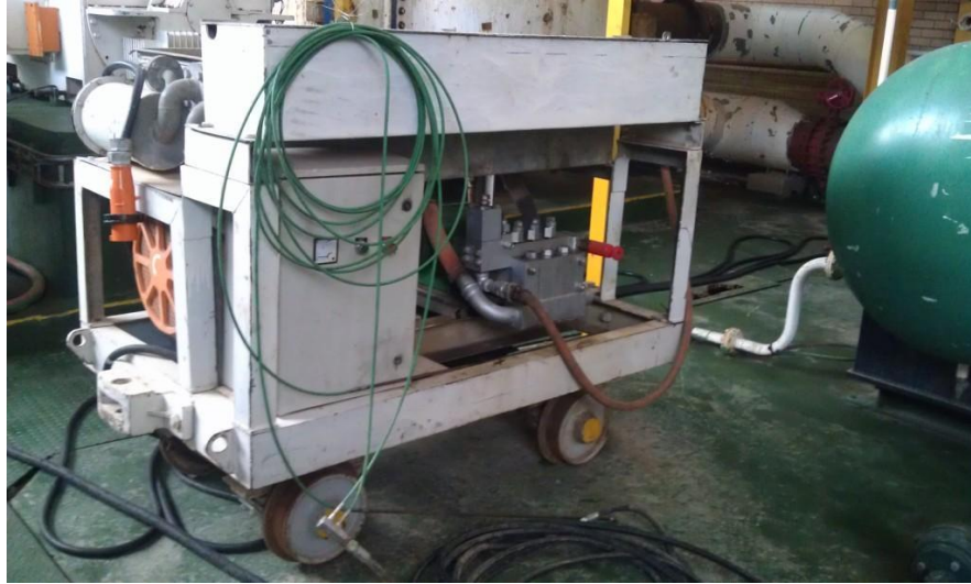
Figure 9: Pressure washer used for cleaning chiller tubes
