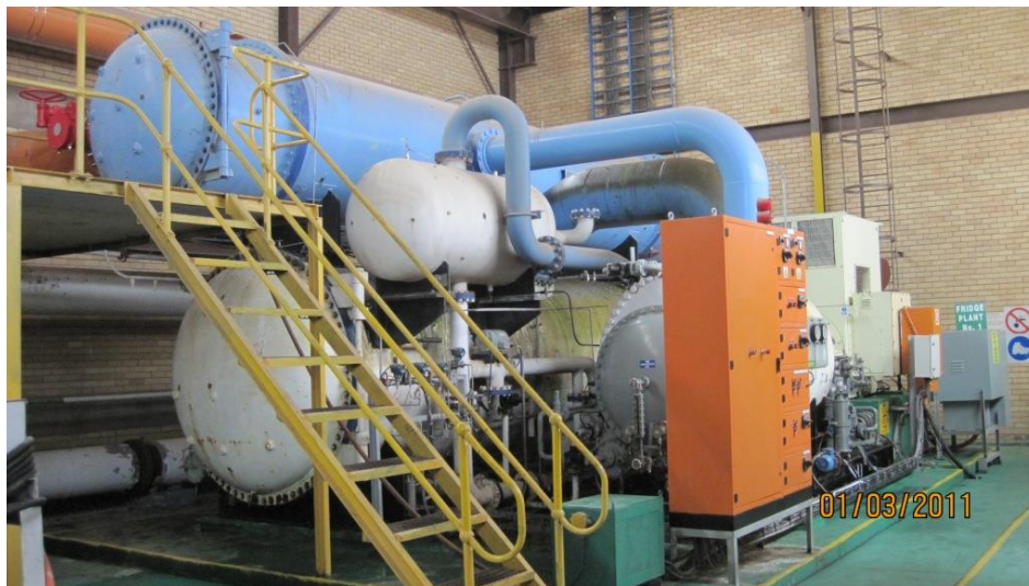
Figure 33: Example of a chiller currently being used on the mine
