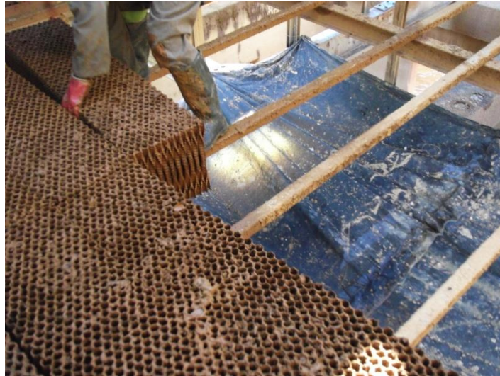
Figure 39: Fill replacement in pre-cooling tower due to excessive sedimentation build up
