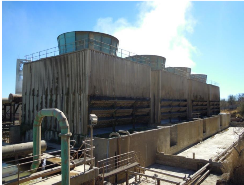
Figure 35: Condenser cooling towers
