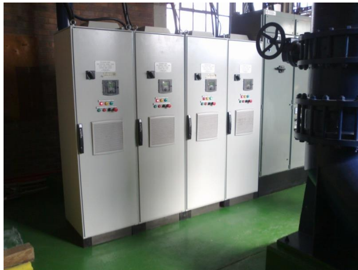
Figure 23: VSDs installed on a mine cooling system
