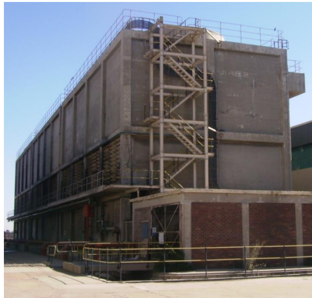
Figure 14: Condenser cooling towers installed on a mine near Klerksdorp
