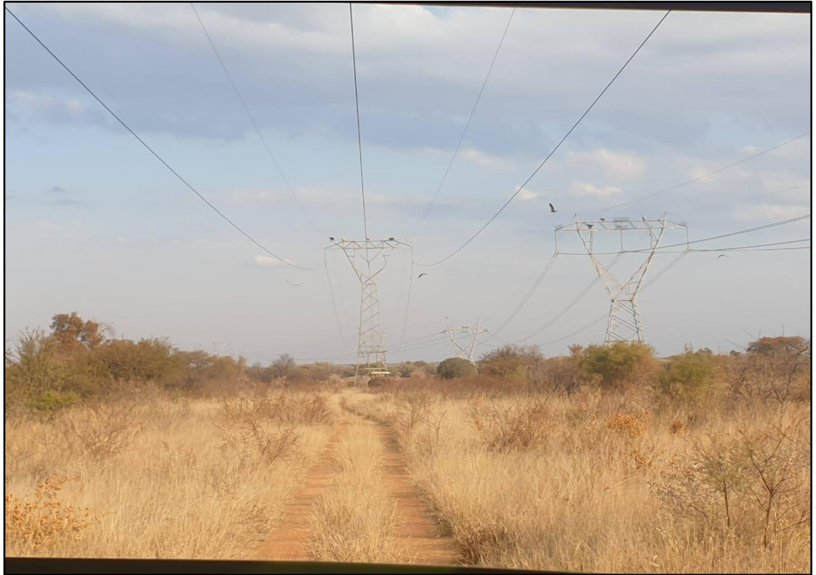
Figure 6-1: Pylons crossing a Limpopo section inside northern DGR. By permission of photographer, Catherine Prinsloo, on 2020-06-16.
