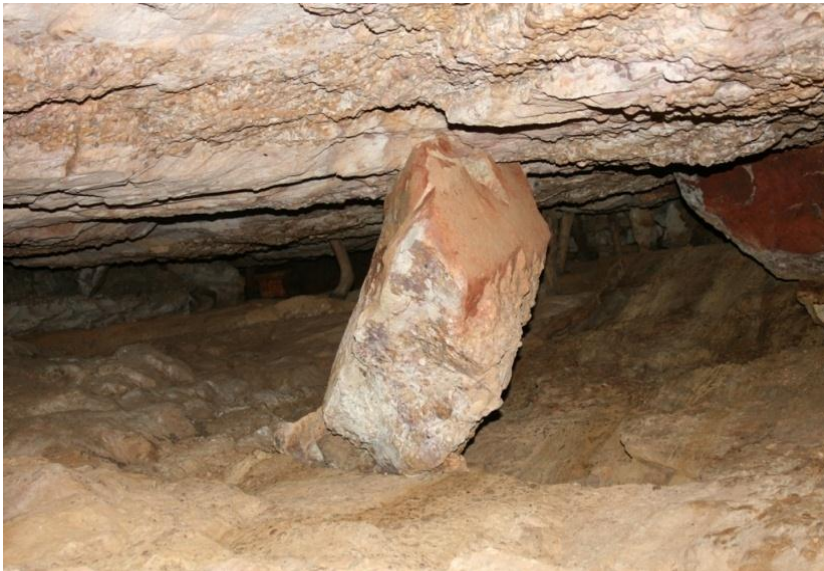
Figure 58. The same stope as in Figure 57, showing signs of collapse and crumbling pillars.
