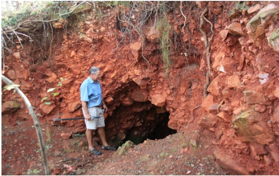
Figure 25. The adit, KL1, on the Red Reef at Koedoeslaagte 516IQ. Note the dangerous condition of the overhang.
