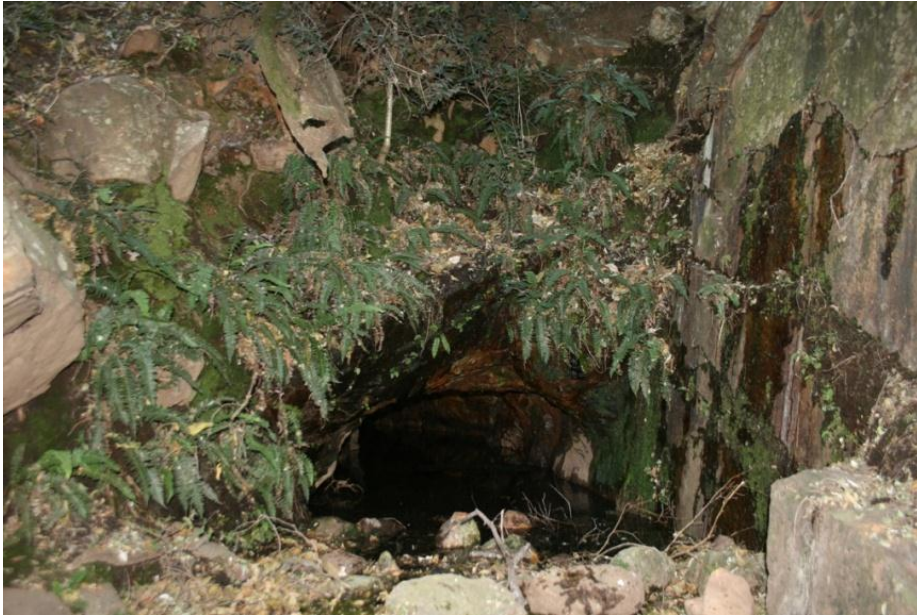
Figure 13. Adit, B8, with dangerous overburden and filled with water on the eastern portion of Buffelskloof 511IQ.
