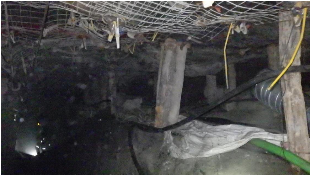
Figure 48: Lack of brattices in a centre gully in an underground working area
