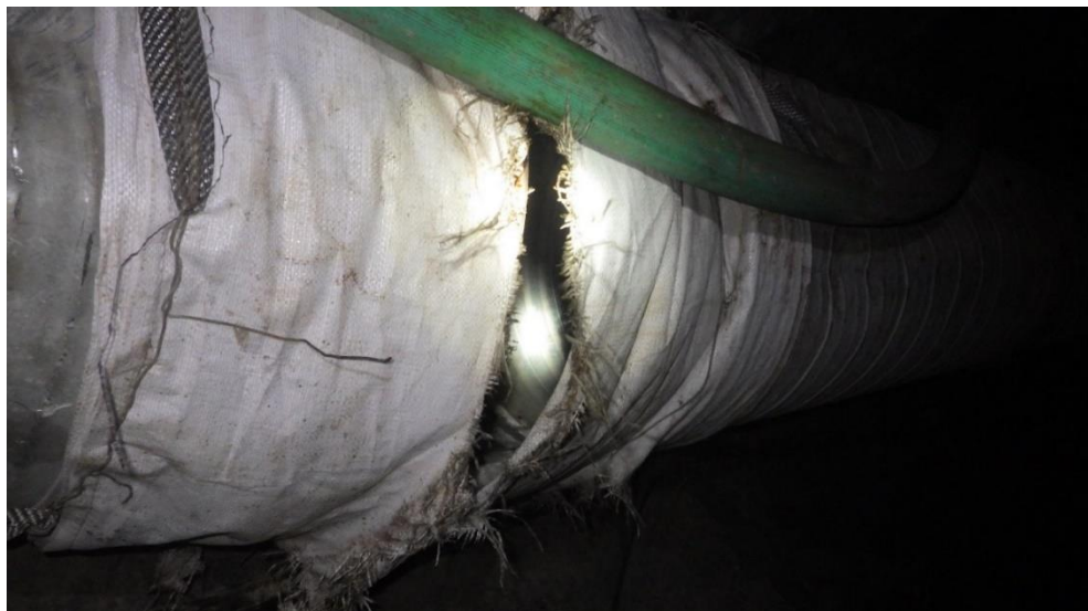
Figure 49: Broken ventilation ducting guiding ventilation air to the working areas
