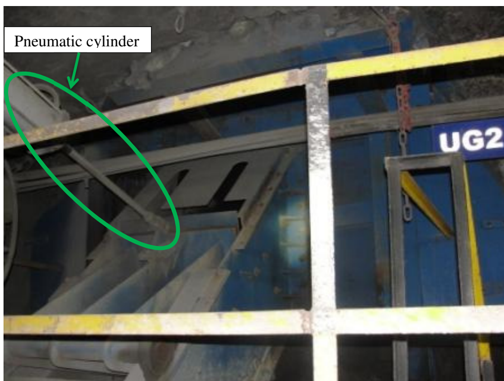
Figure 6 – Pneumatic cylinder installed on a loading box 8
