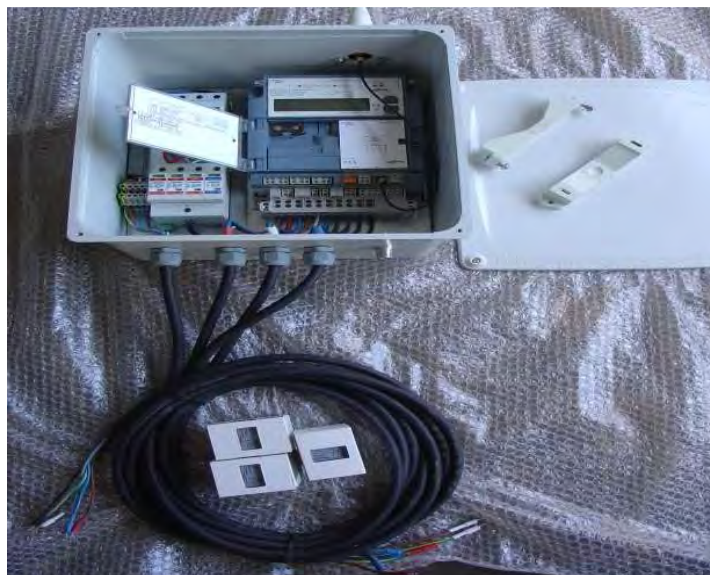
Figure 4-9: Logger kit comprising meter, surge arrester, circuit breaker, box cover with brackets, CT cables and three CTs
