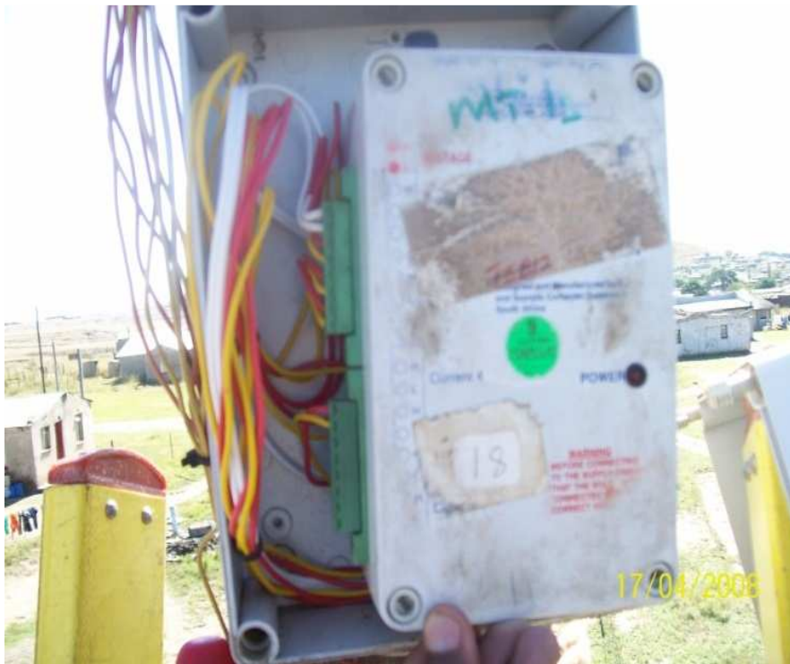
Figure 4-8: Installed old logger showing wires connecting the current transformer (CT)
