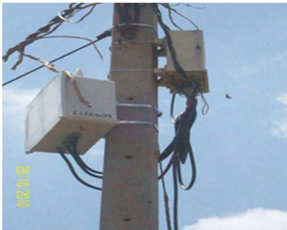
Figure 4-12: Logger installed on a concrete pole
