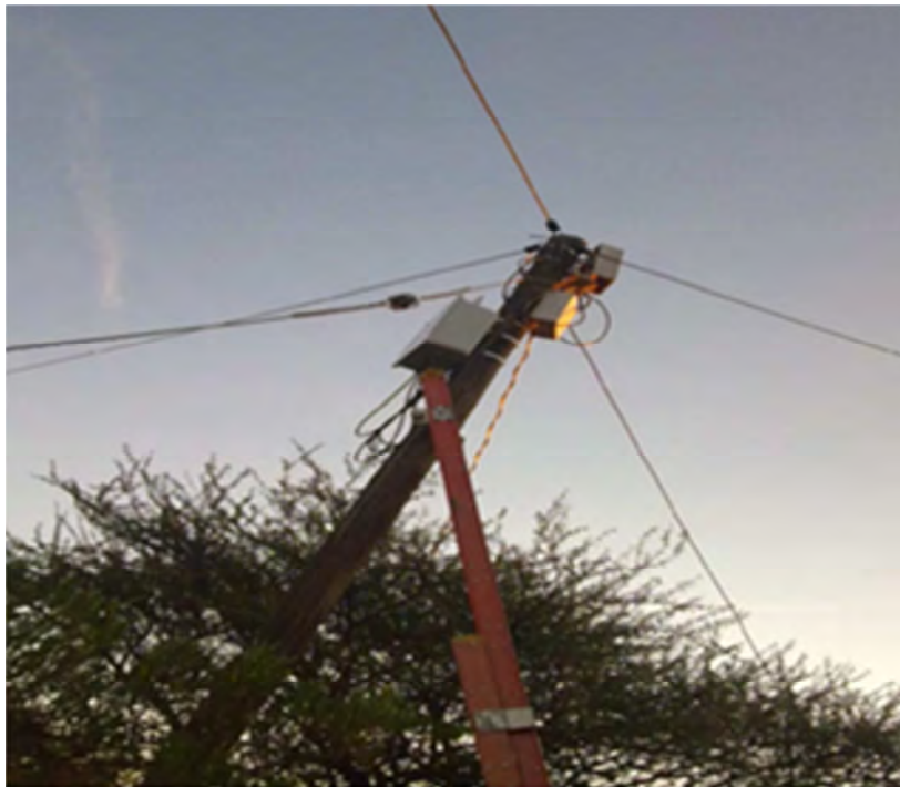
Figure 4-11: Logger installed on a wooden pole
