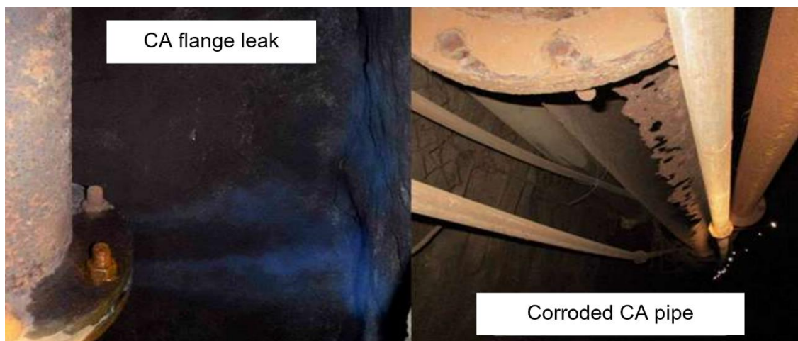
Figure 11: CA leak on a pipe flange and a corroded CA pipe [8]
