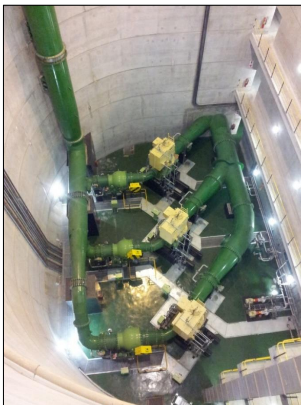
Figure 38: Low-lift pump station well with 3 pumps
