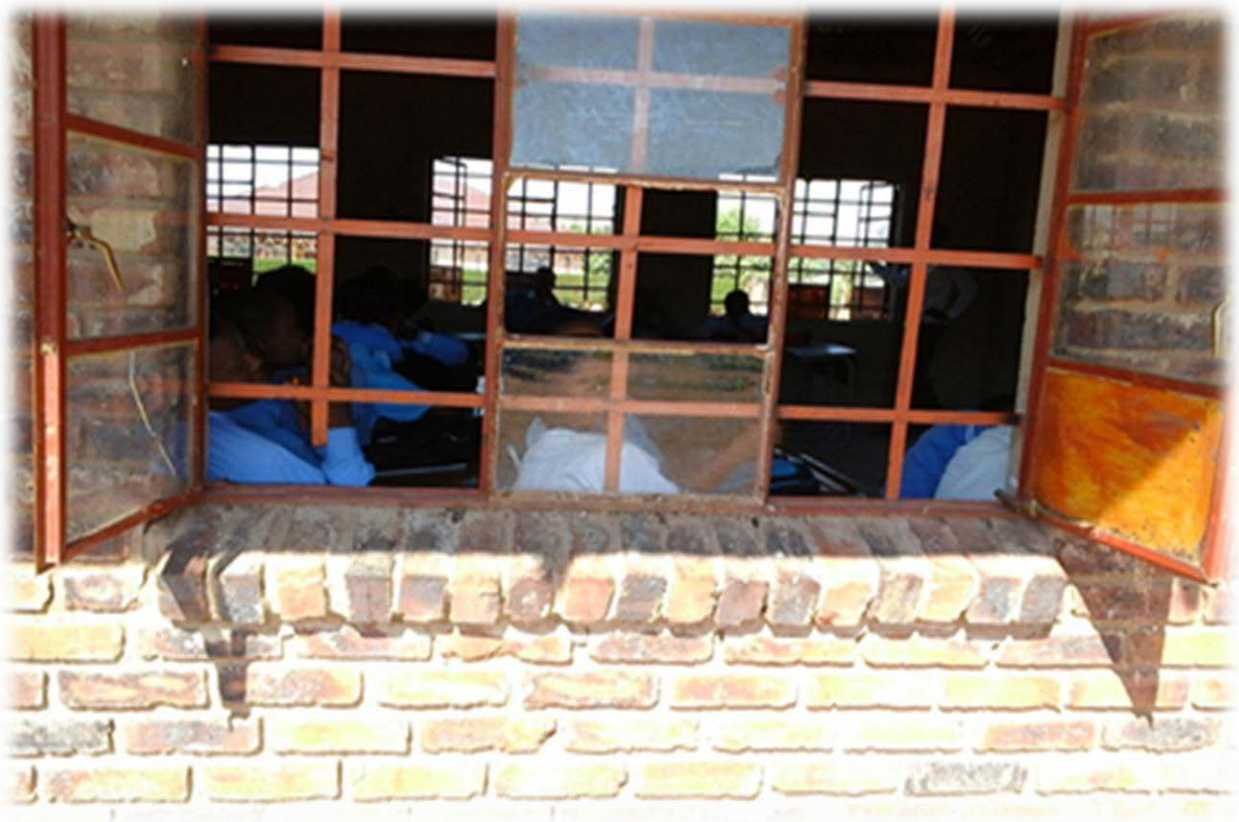
Figure 5-4 Some window panes either broken or have fallen out
