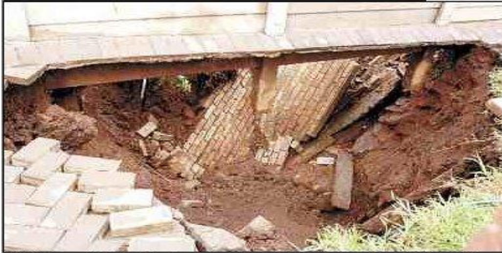
Misfortune: This is all that remains of one Centurion townhouse's foundation after a sinkhole damaged most of the property. Photo: Herbert Matimba, Pretoria News
