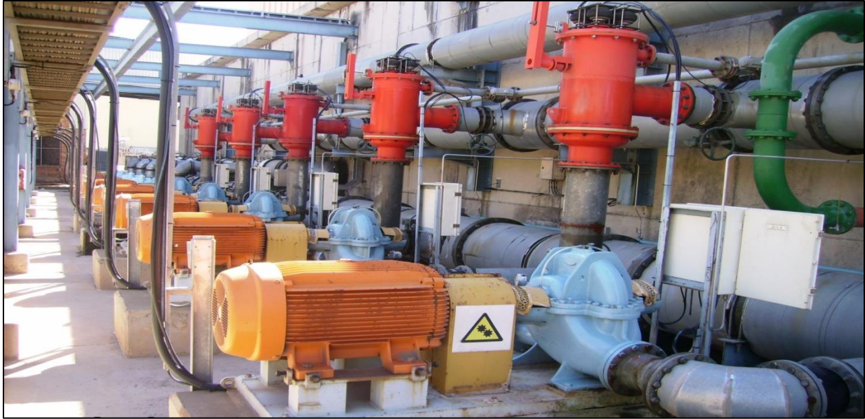
Figure 3 - 7: Evaporator pumps of Mine A surface cooling system 6
