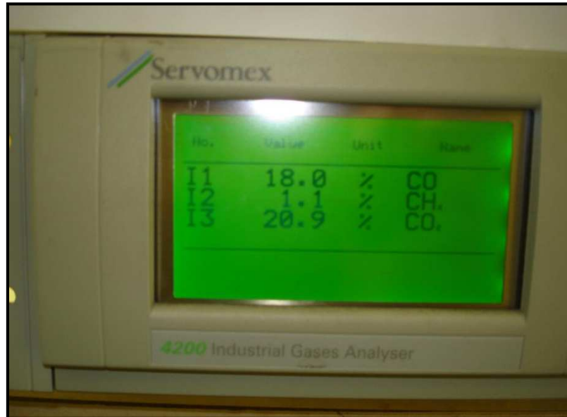
Figure D.1.17: Servomex infrared gas analyser
