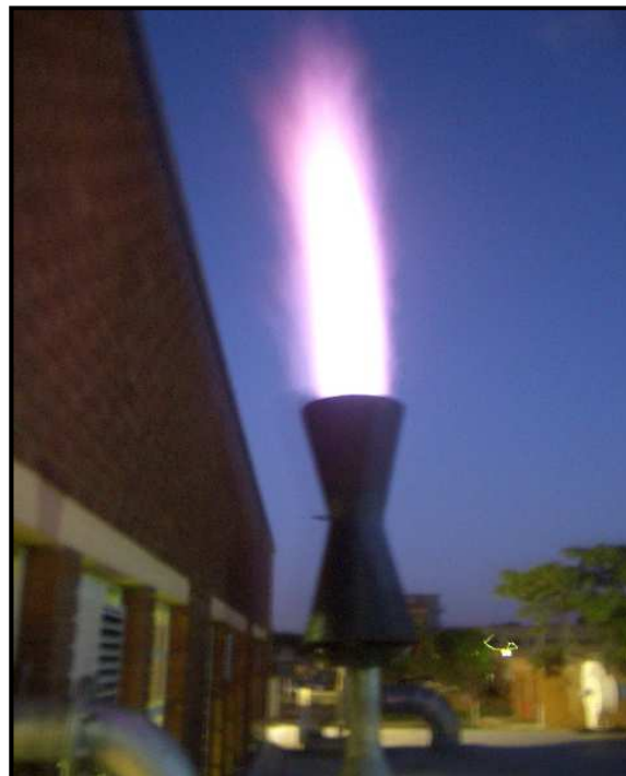
Figure 4.14: Flaring of gas produced by the fluidised bed gasifier
