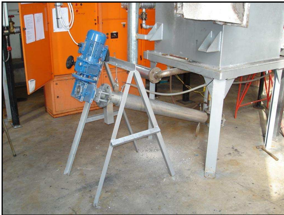
Figure D.1.3: Water-cooled bed char extraction screw conveyor
