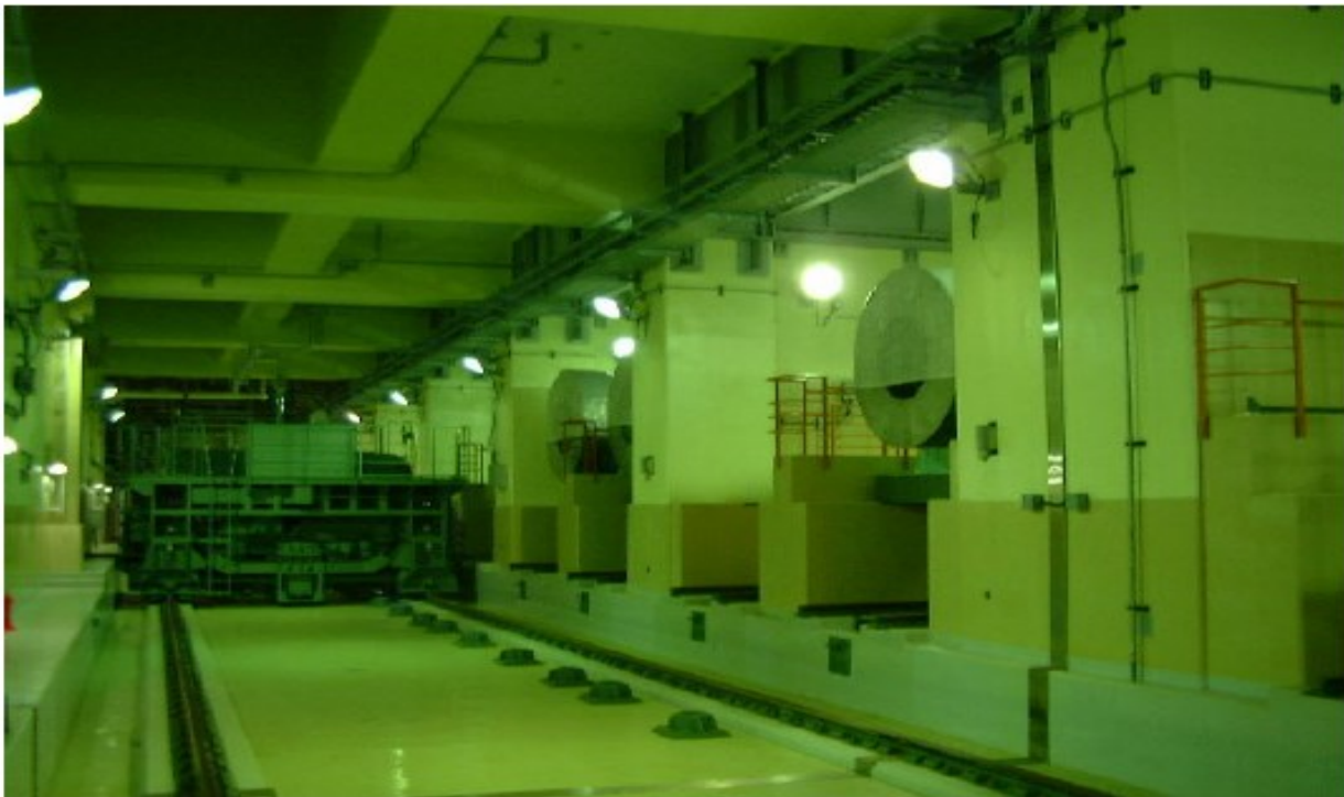
Figure 2-10: Fukushima dry storage facility in Japan (Gilmore, 2018)
