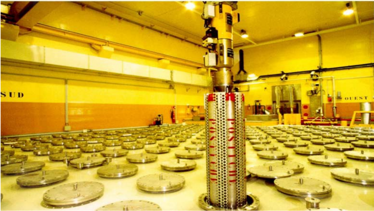
Figure 2-15: Cascad dry vault storage facility (AREVA, 2010)
