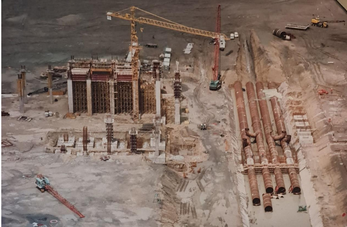
Figure 69: CW ducts being constructed below the turbine hall of a fifth-generation power station
