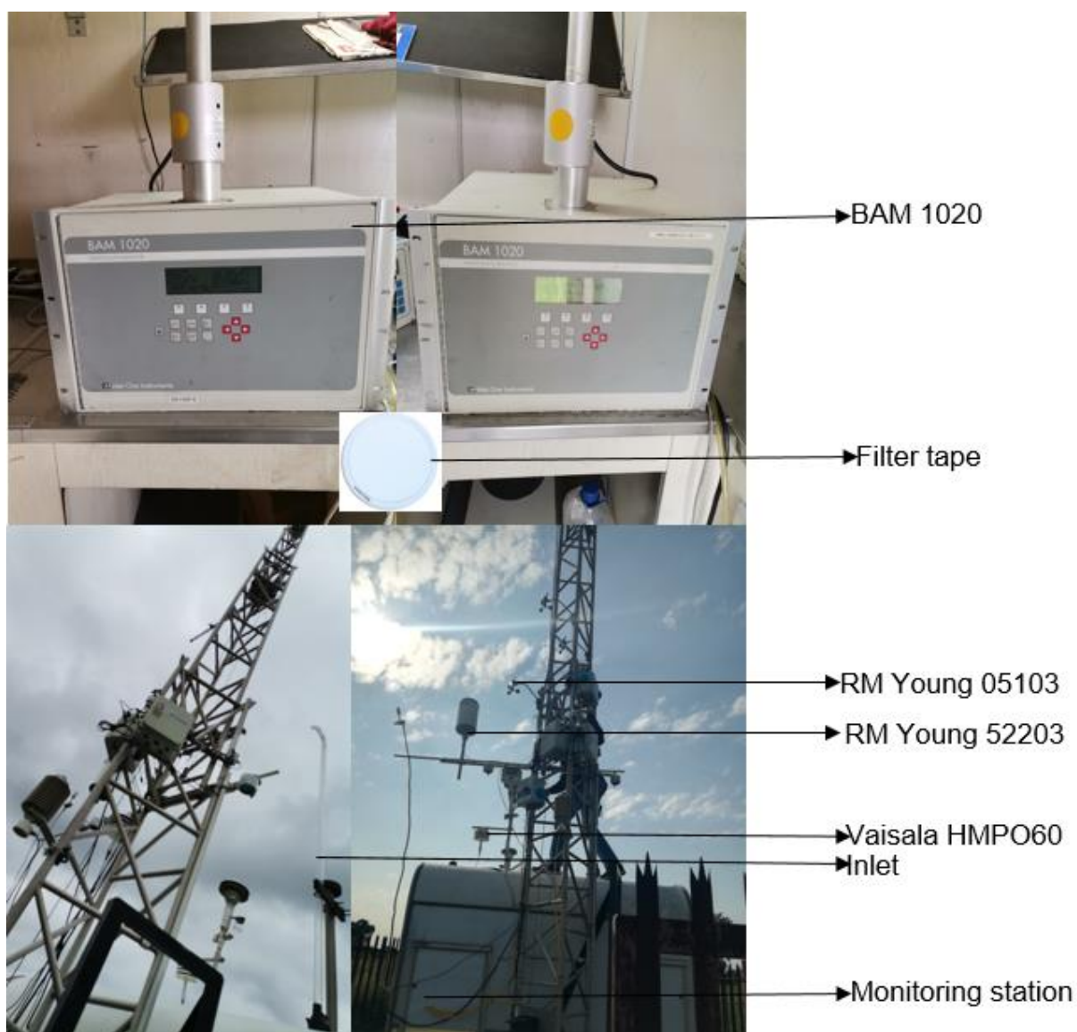
Figure 3-4: Fixed monitoring station in Zamdela showing PM and meteorological analysis used during the sampling campaign
