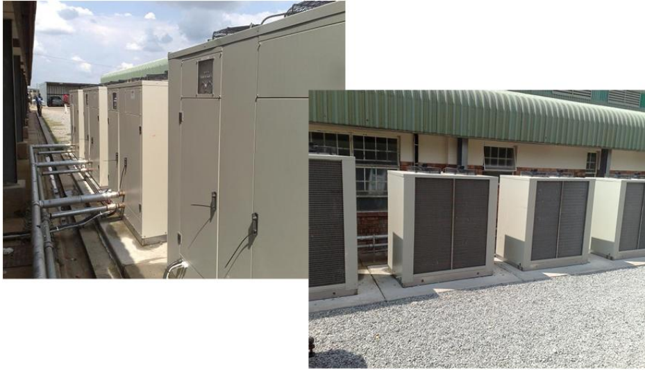
Figure 2.1: South African industrial heat pump installation utilizing R407c (van Eldik 2012).
