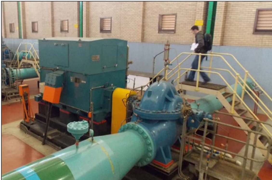
Figure 10: Single stage double suction horizontal centrifugal pumps (photo by author)
