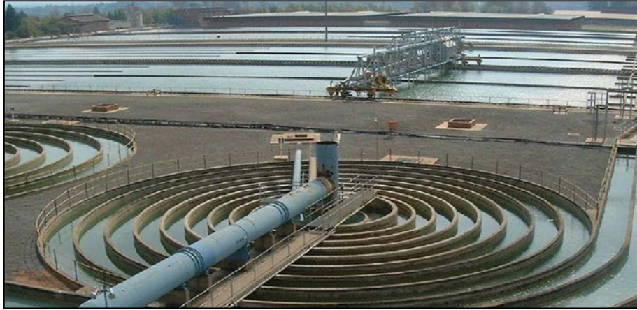
Figure 21: Clarifier and flocculator at a WTW [19].
