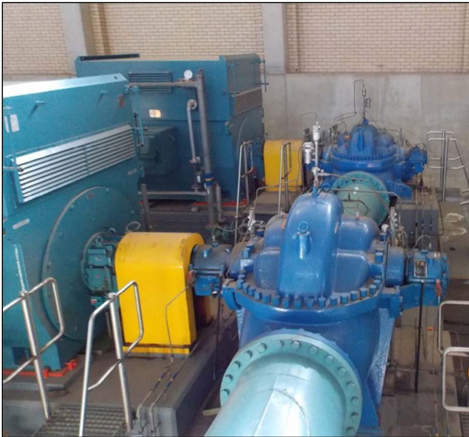
Figure 9: Double stage double suction horizontal centrifugal pump set (photo by author)
