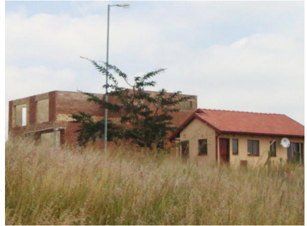
Figure 48: A larger bonded unit being constructed next to a smaller bonded unit
