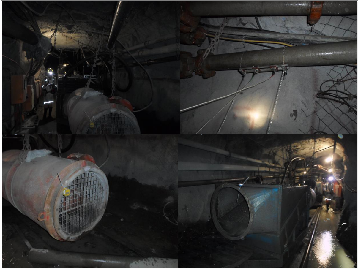
Figure 124: Manual measurements on MCUs and PRVs – Mine A
