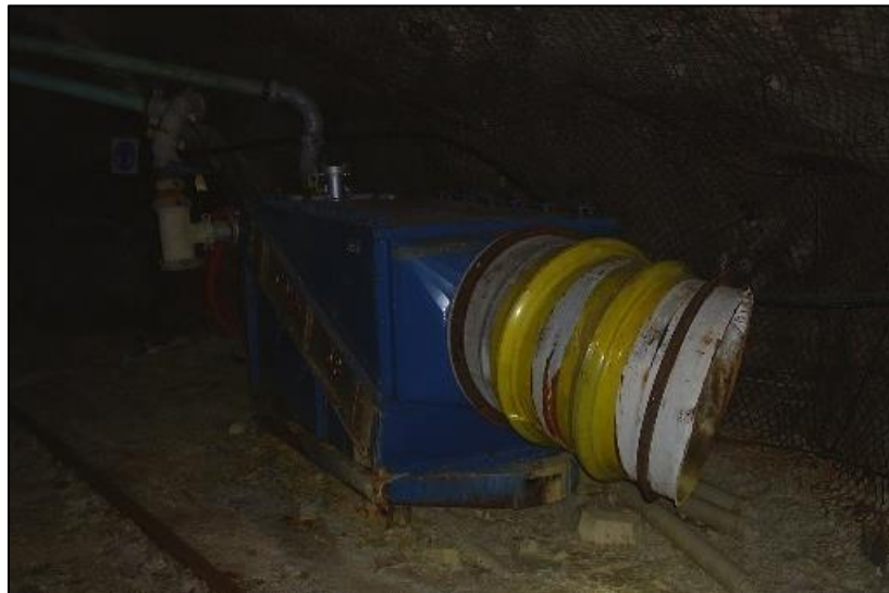
Figure 113: Mobile spot cooler situated underground
