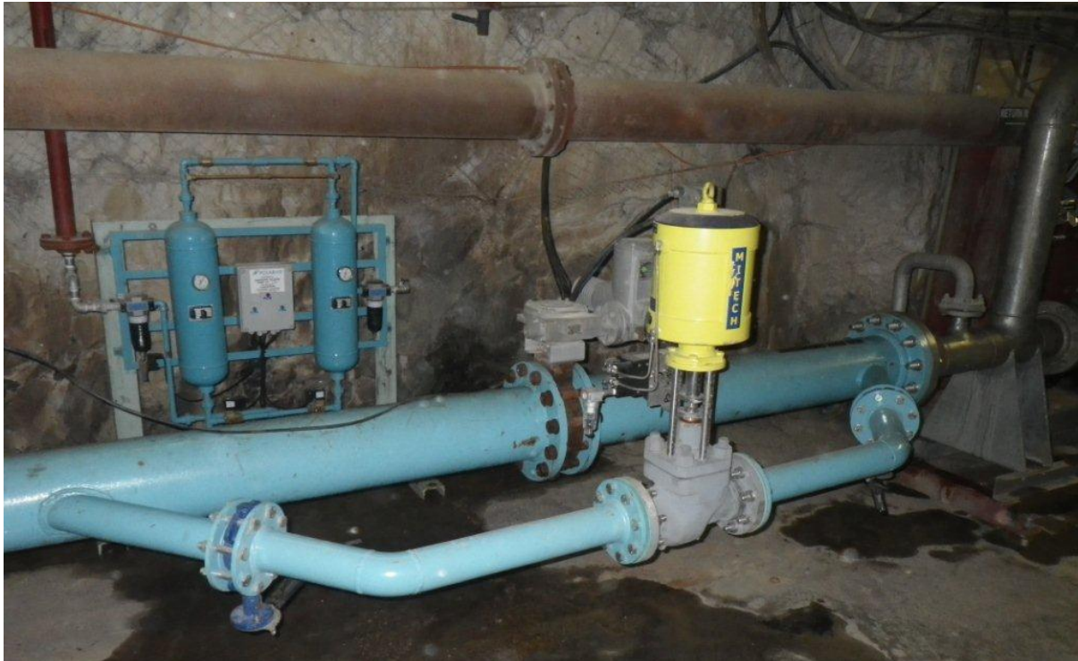
Figure 111: WCS installed at a deep-level gold mine – 2 km deep
