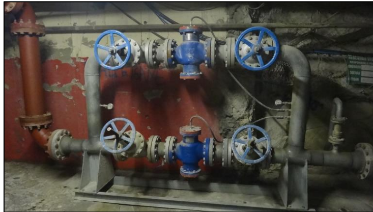
Figure 106: Pressure-reducing station situated on a mining level
