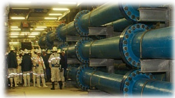
(b) 3CPFS installed at a mine
