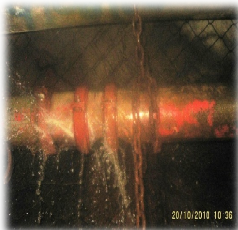
(a) Leaking pipes
