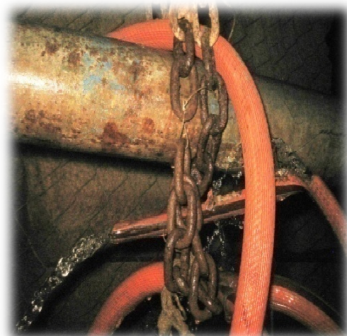
(b) Unattended water hoses
