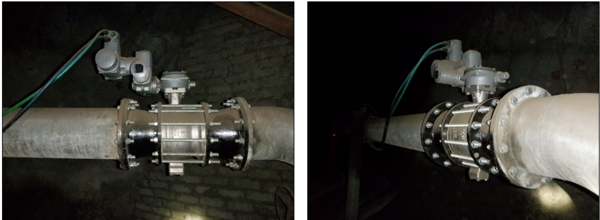
Figure 50 - Segmented V-notch ball valve installed on 25 level at Shaft A.
