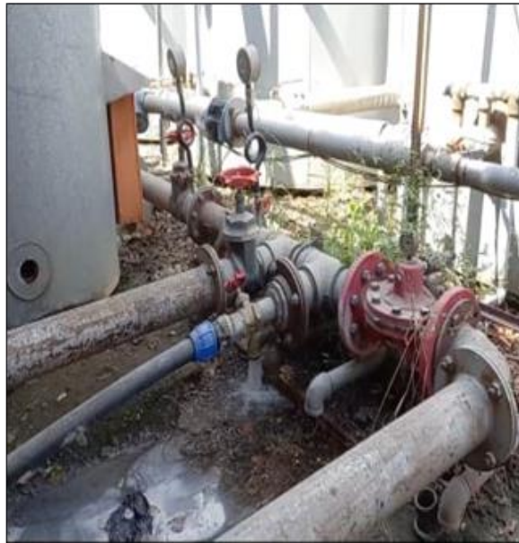
Figure 59: Photo of leak found at the geyser
