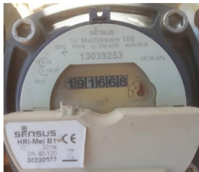
Figure 22: Photo of mechanical flow meter
