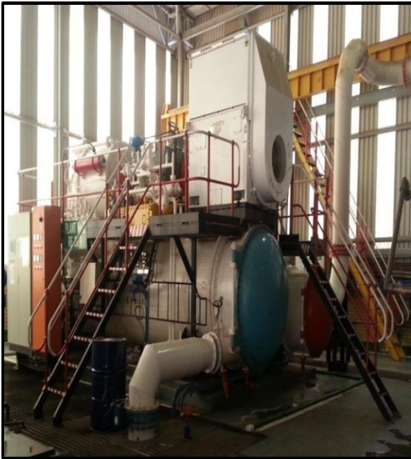
Figure 1-6 : Fridge plant on a deep-level gold mine
