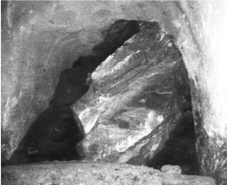
Figure 1-2: A photo of a large rock blocking an ore pass and causing a restriction to the flow of ore and waste rock (Szwedzicki, 2007).
