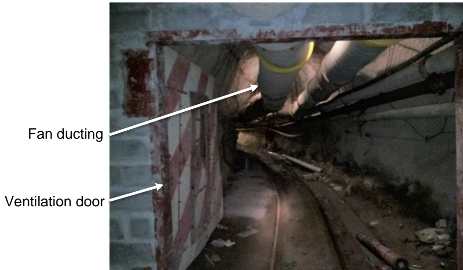
Figure 1-5: Crosscut entry with a ventilation door and regulator 3
