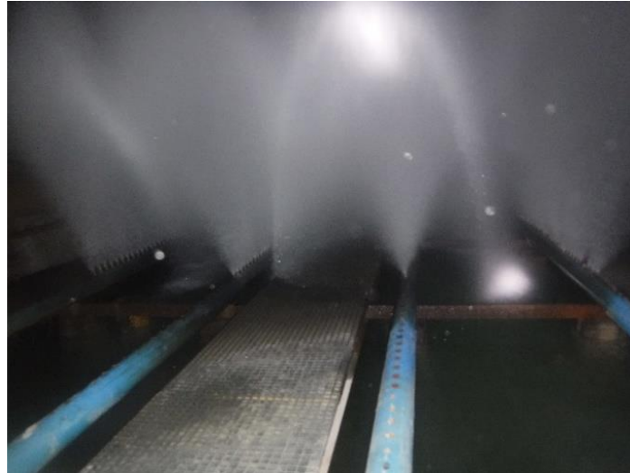
Figure 1-12: Direct contact heat exchanger used underground
