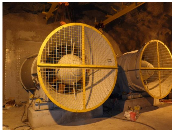
Figure 1-8: Booster fan located underground to provide airflow [14]
