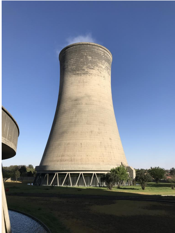
Natural Convection Cooling Tower
