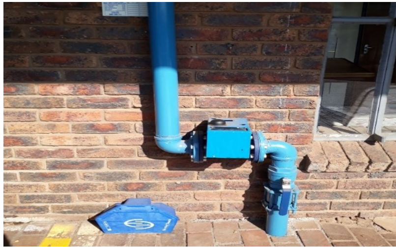
Figure 5.33: Node at Building-36
