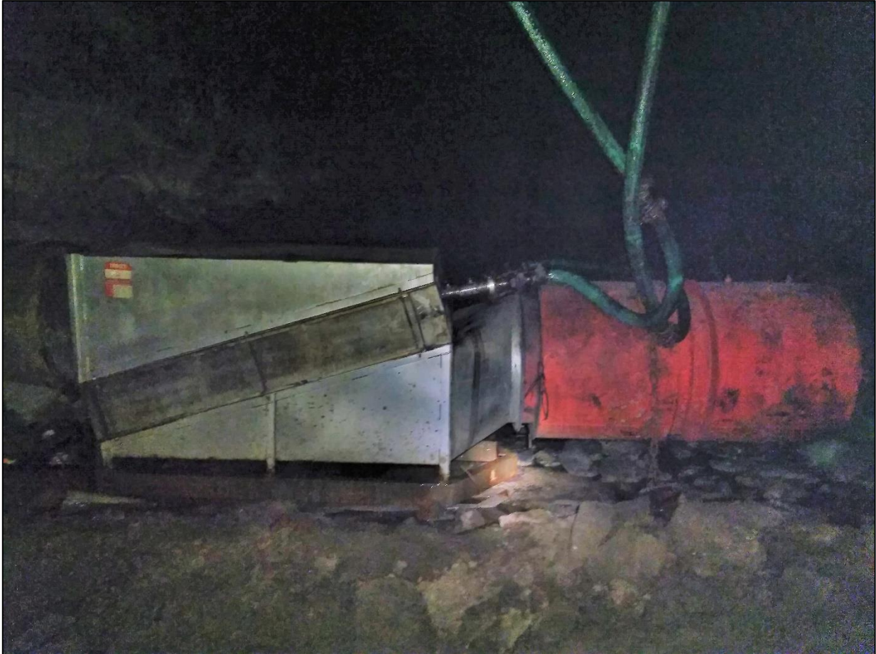
Tertiary cooling - Underground cooling coil xxx
