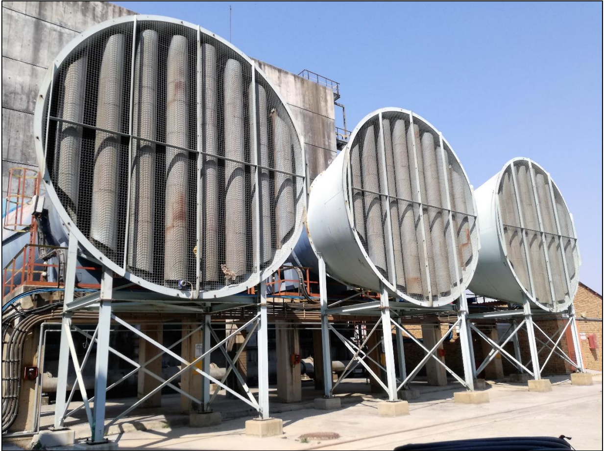
Primary cooling - Surface bulk air coolers vii
