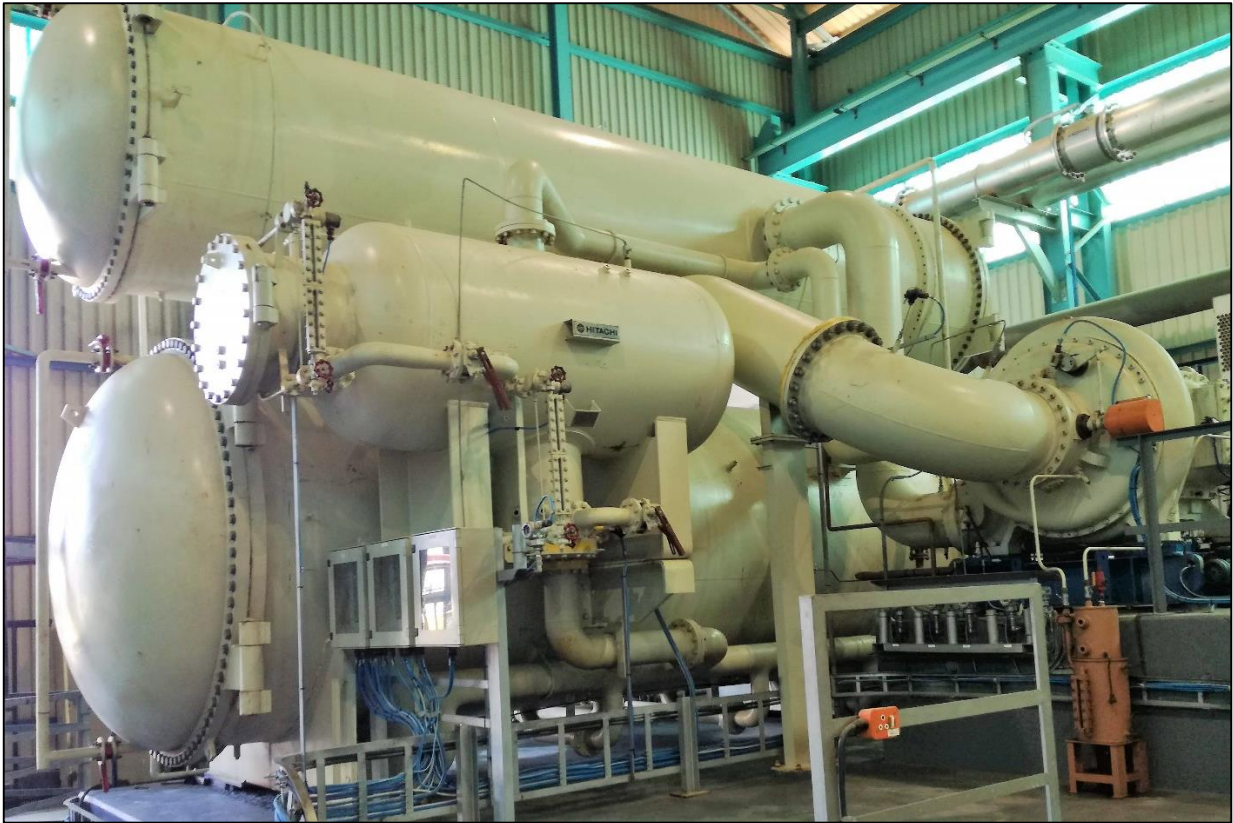
10 MW Surface Fridge Plant i
