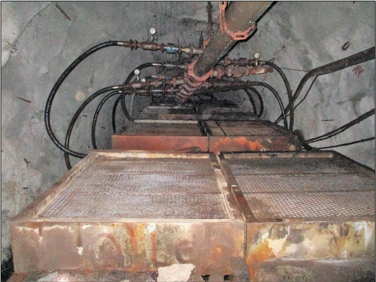
Secondary cooling – Underground bulk air cooler xvii
