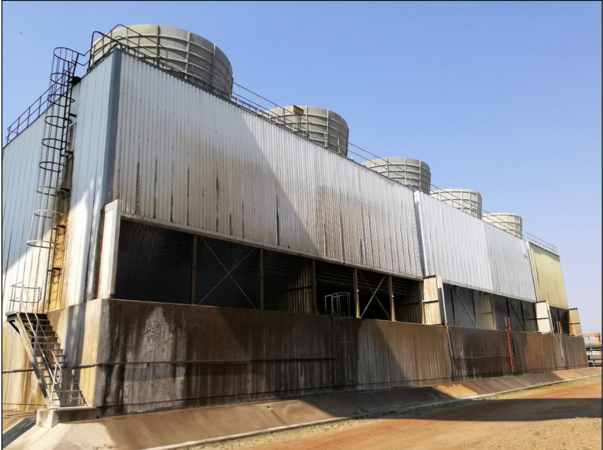
Heat rejection – Surface cooling towers xxxii
